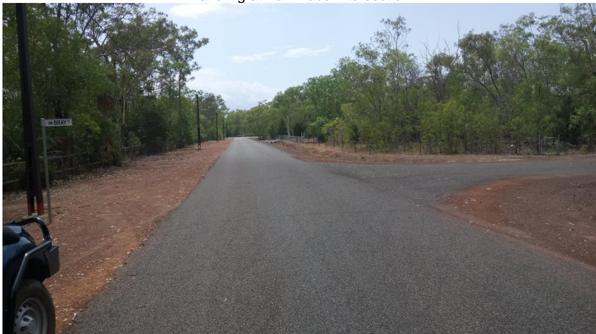
Raveling at Bray Place Intersection
