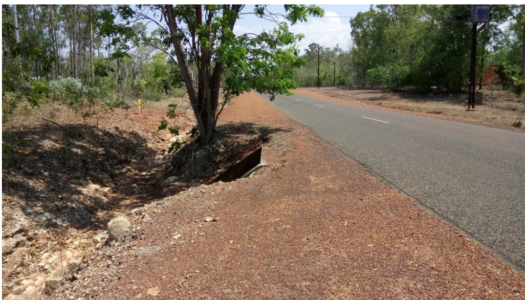
Photo: Unprotected Culvert Erickson Crescent
