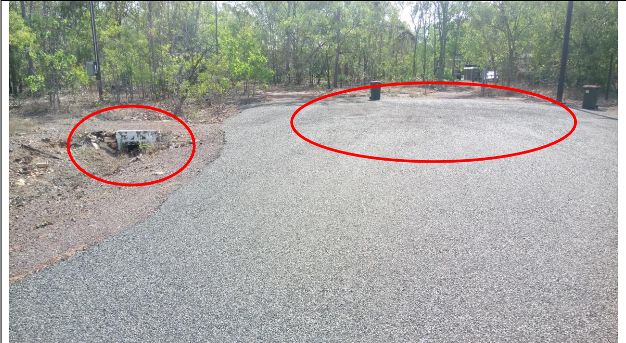
Ravelling and unprotected drainage structure at Boom Place cul-de-sac
