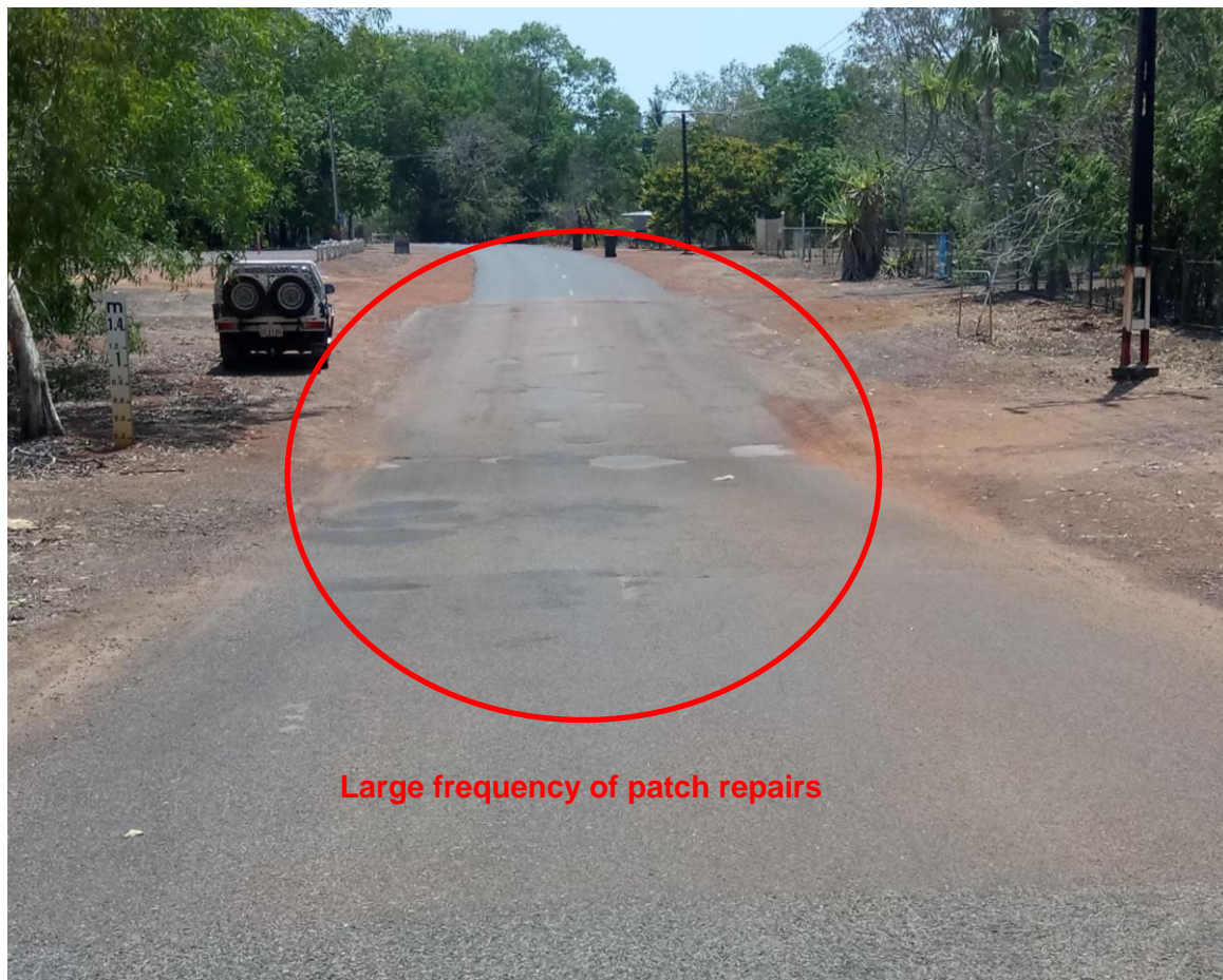
Figure 4 – Road section of maintenance concern, 92 Cox Drive
