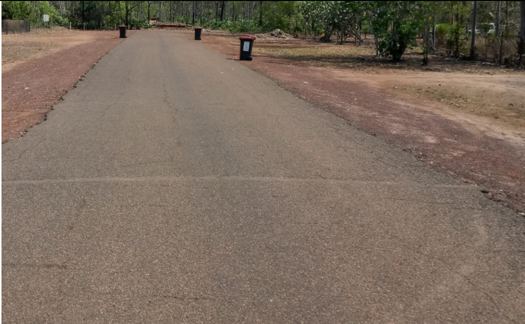
Cracking between CH0.0-CH0.1
