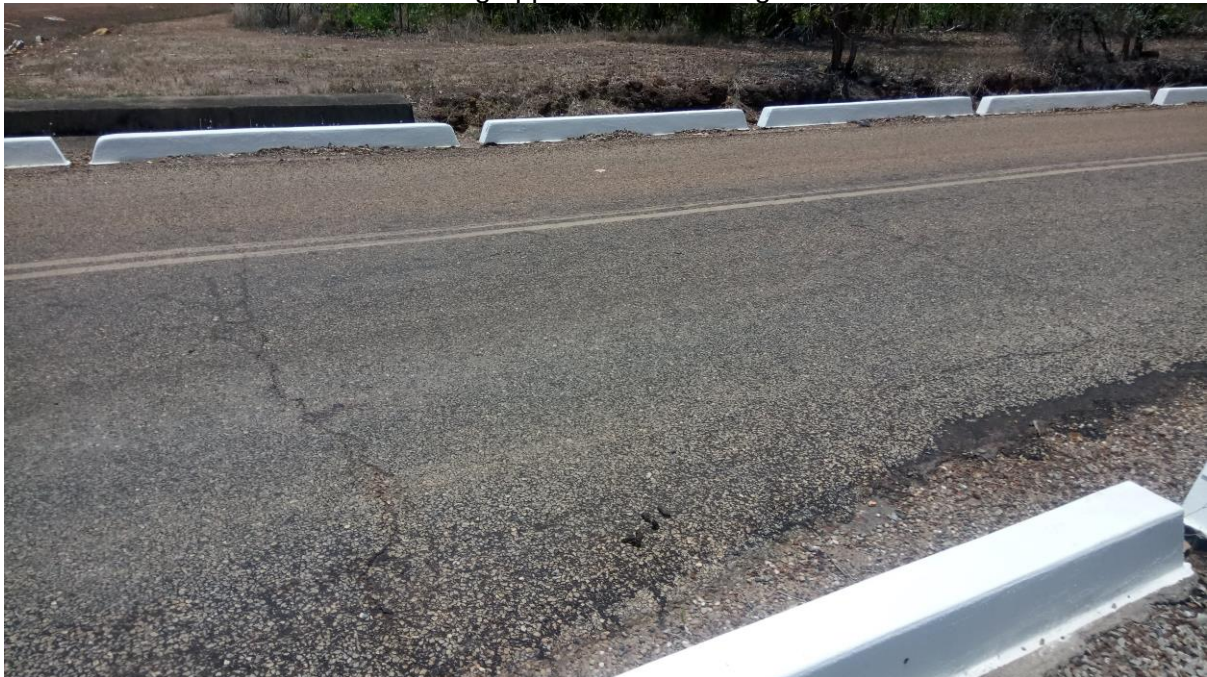
Cracking at Cox Drive intersection
