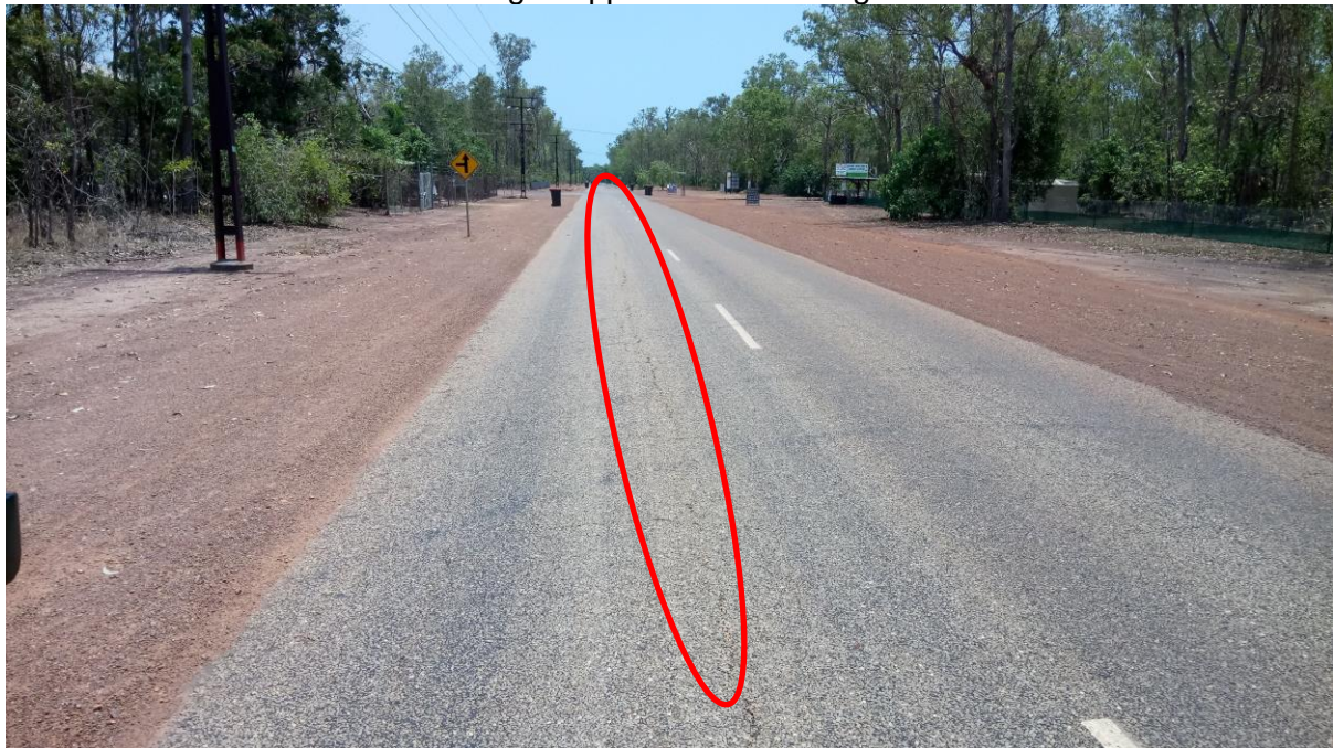
Cracking at approximate chainage 0.5
