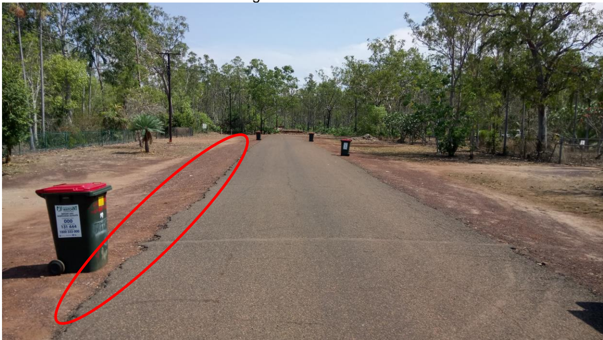
Edge break between CH0.0-CH0.1
