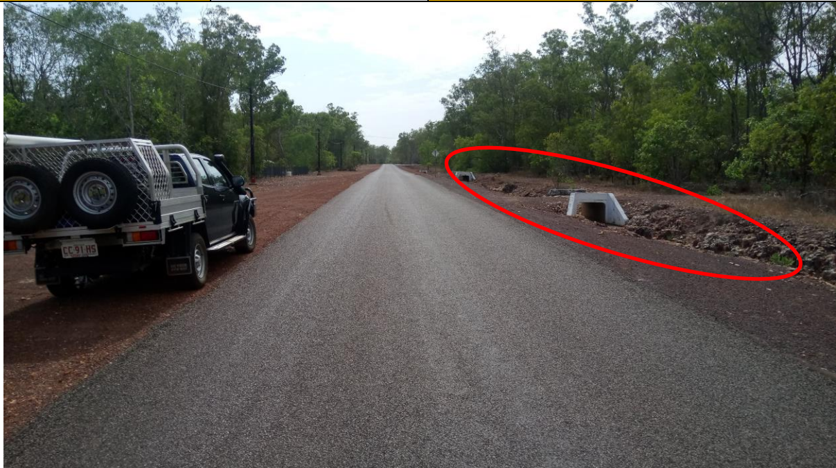
Unprotected culverts at approximate chainage 0.1
