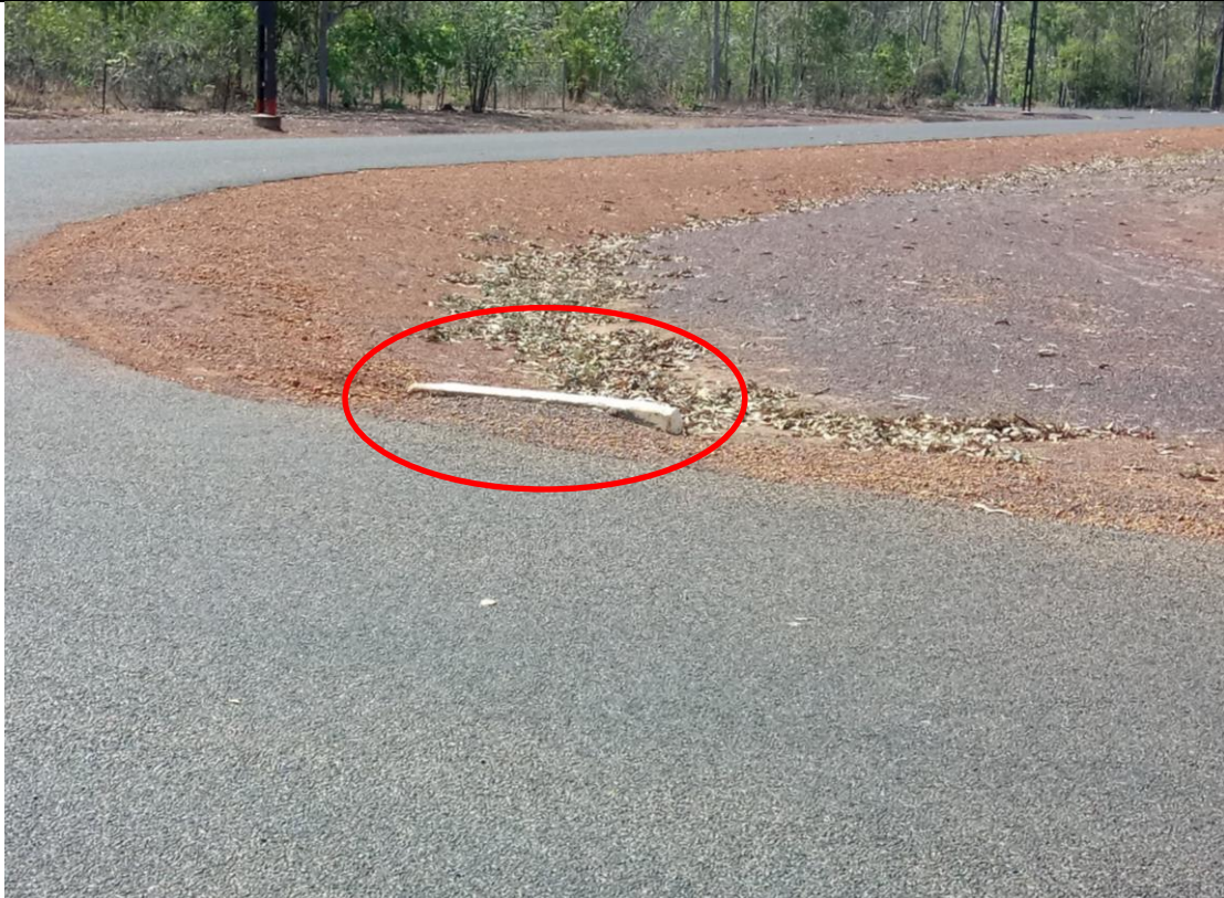
Unprotected Drainage Structure Dalmeny Street Intersection
