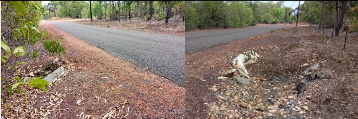
Unprotected culvert at approximate chainage 0.05
