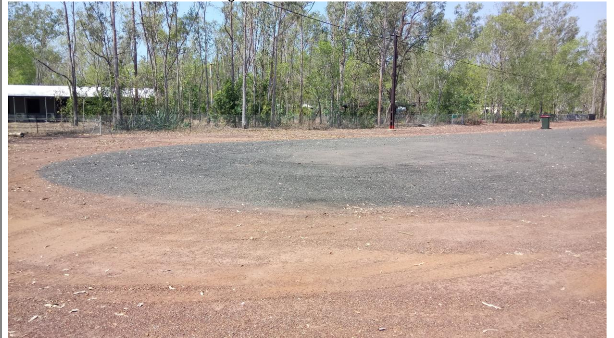
Raveling at Cul-de-sac
