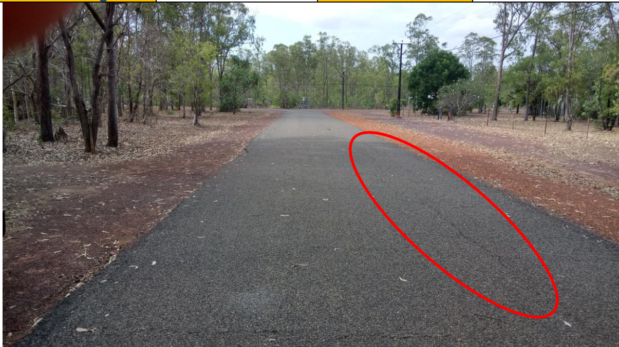
Cracking at approximate chainage 0.3
