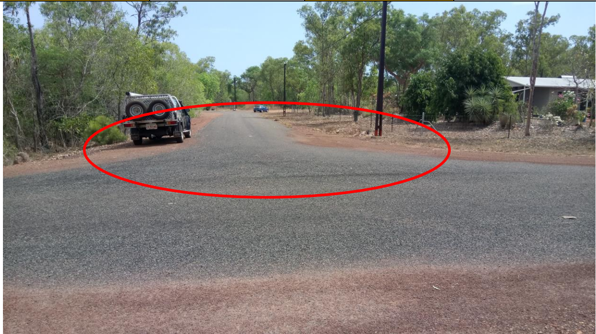
Raveling at Harney Street Intersection
