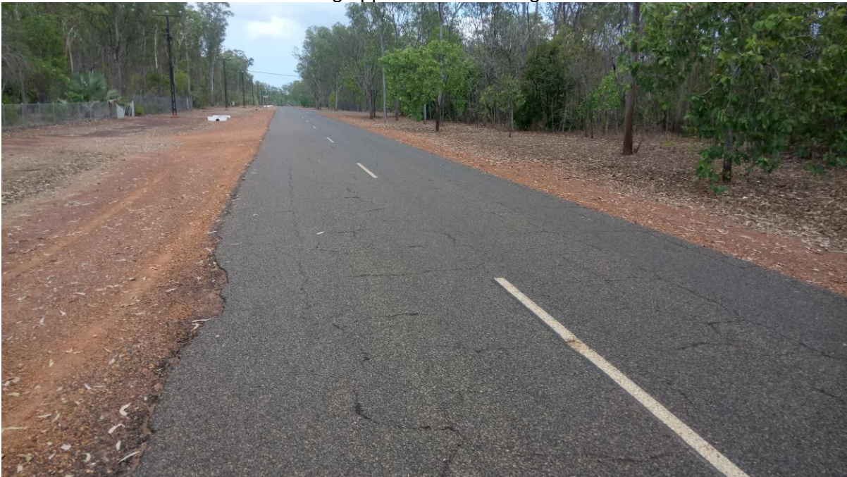
Cracking approximate chainage 1.6
