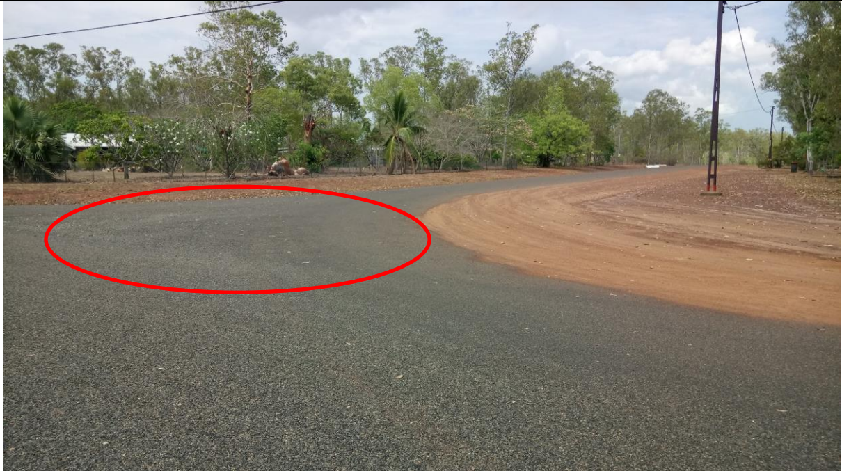
Raveling at Milady Street Intersection
