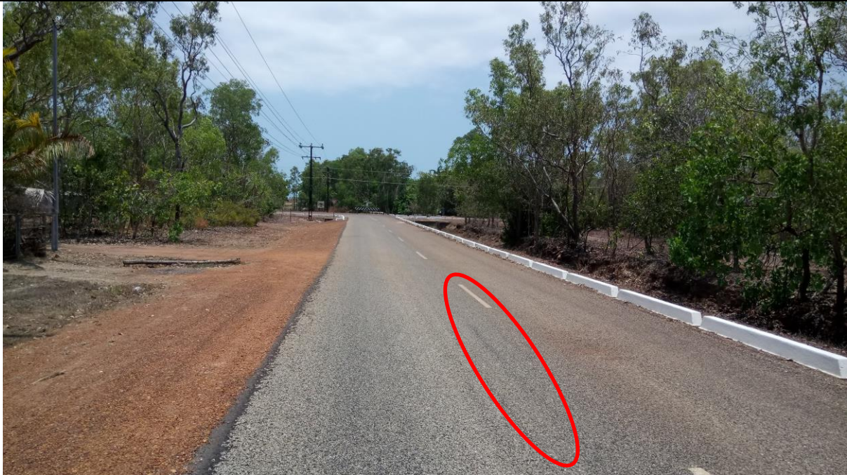
Cracking approximate chainage 1.1
