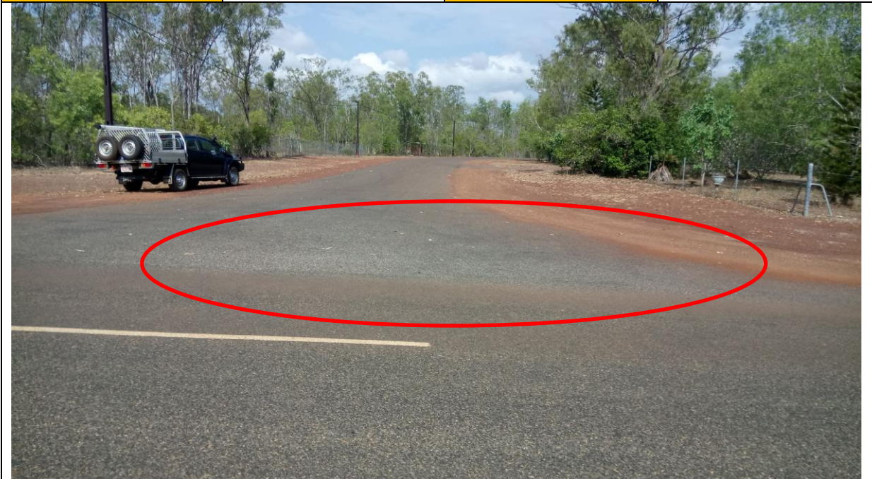
Raveling Erickson Crescent Intersection
