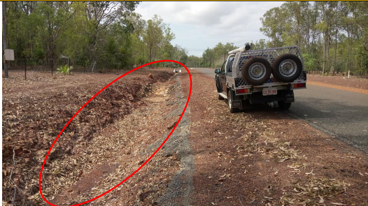
Unprotected open drain and culvert structures approximate chainage 0.1
