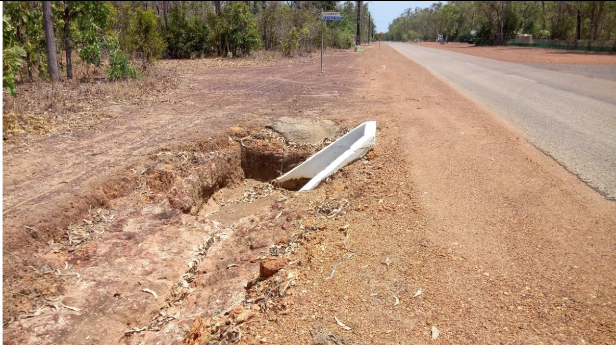
Unprotected culvert at approximate chainage 0.4
