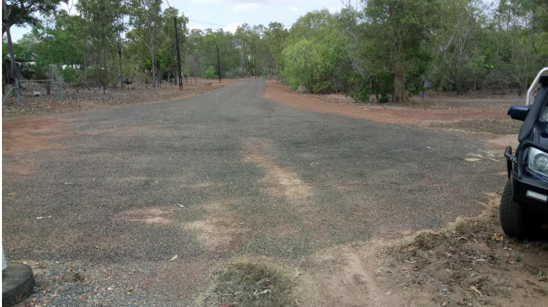
Raveling at Cul-de-sac
