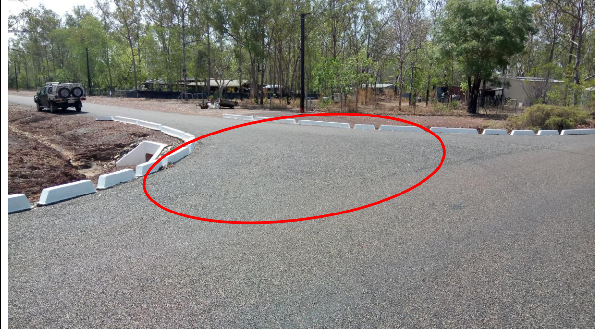
Raveling at Brisbane Street Intersection
