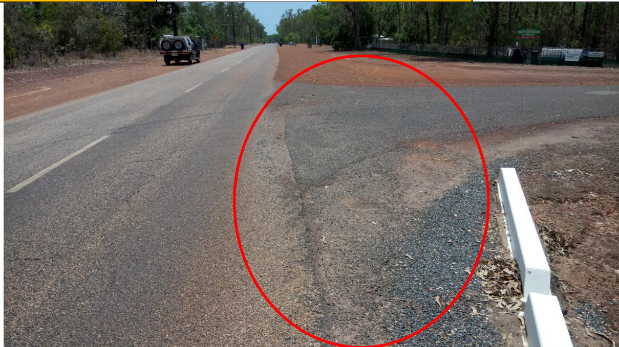
Raveling at Forsyth Road Intersection
