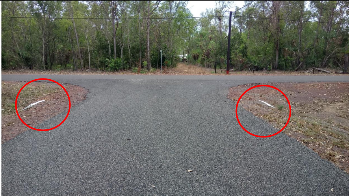
Unprotected drainage structure Uhr Road Intersection
