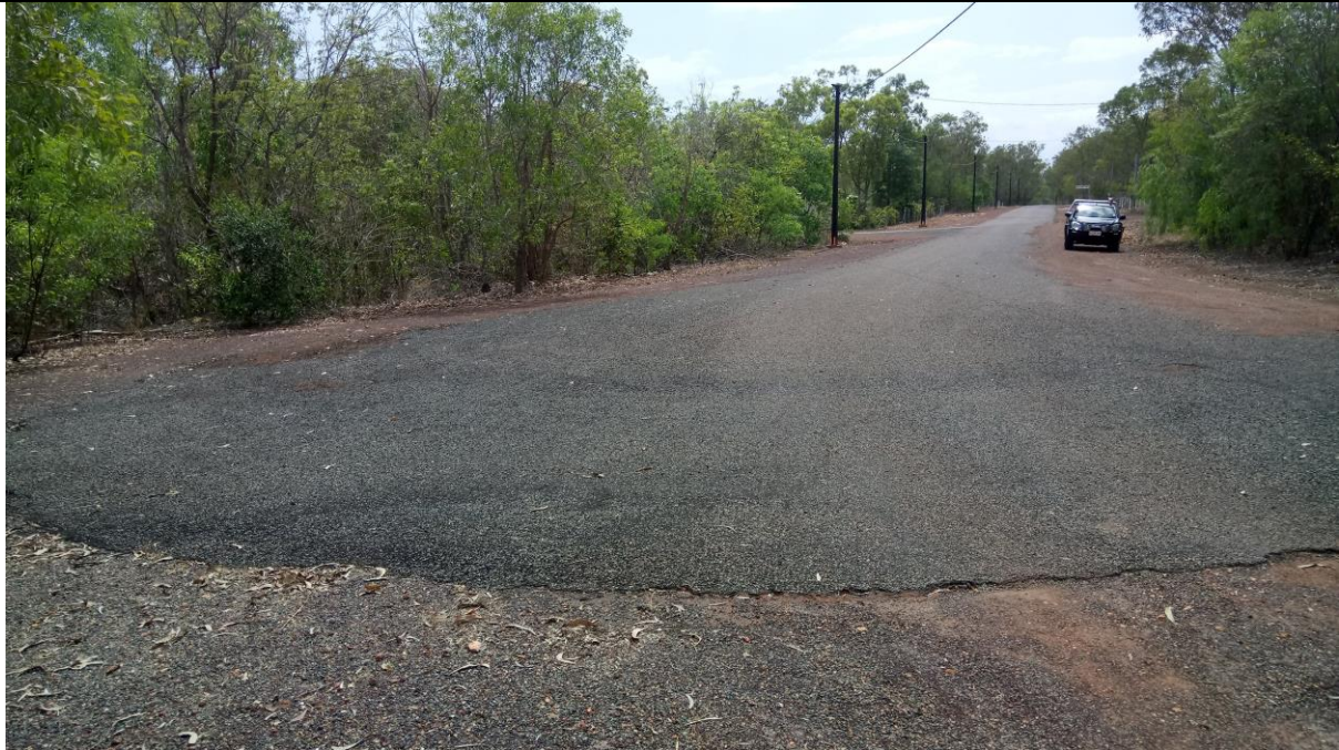
Raveling at cul-de-sac
