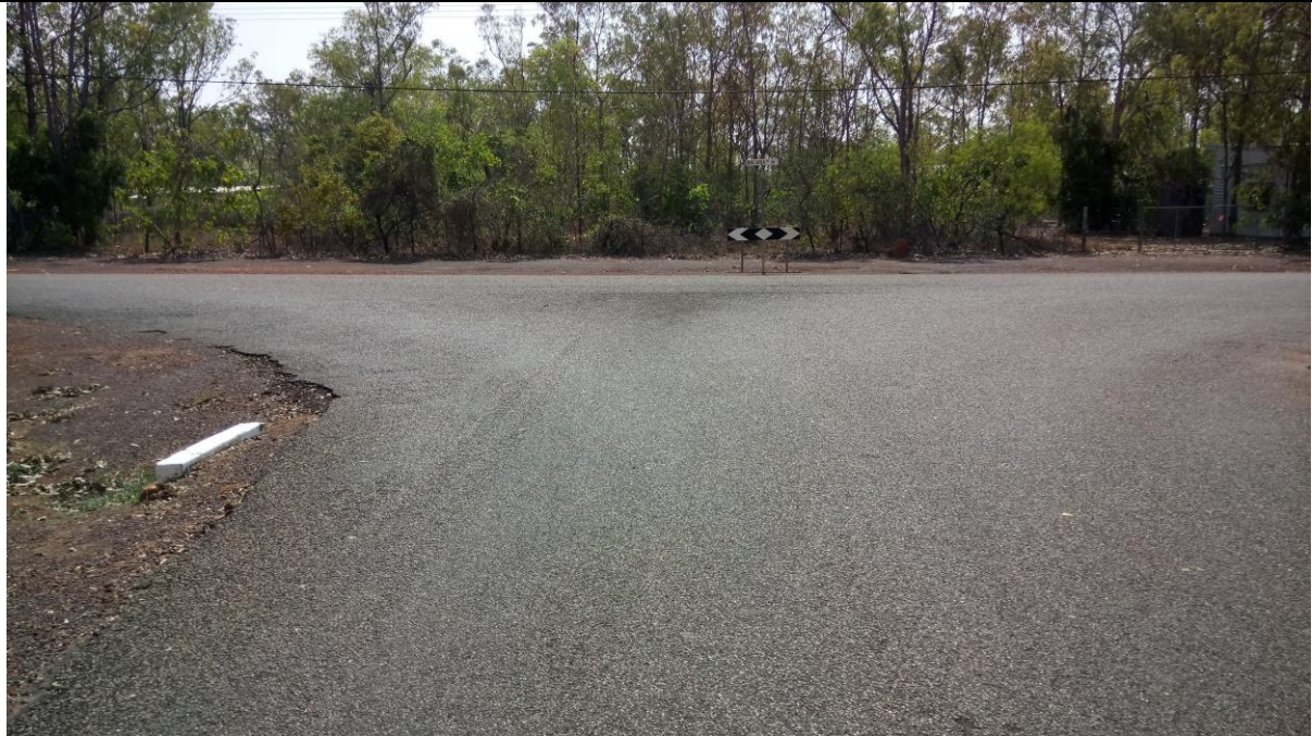
Ravelling at Baluria Road
