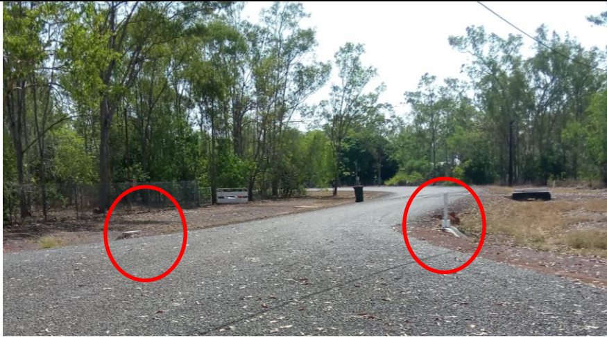
Unprotected Culvert approximate chainage 0.2
