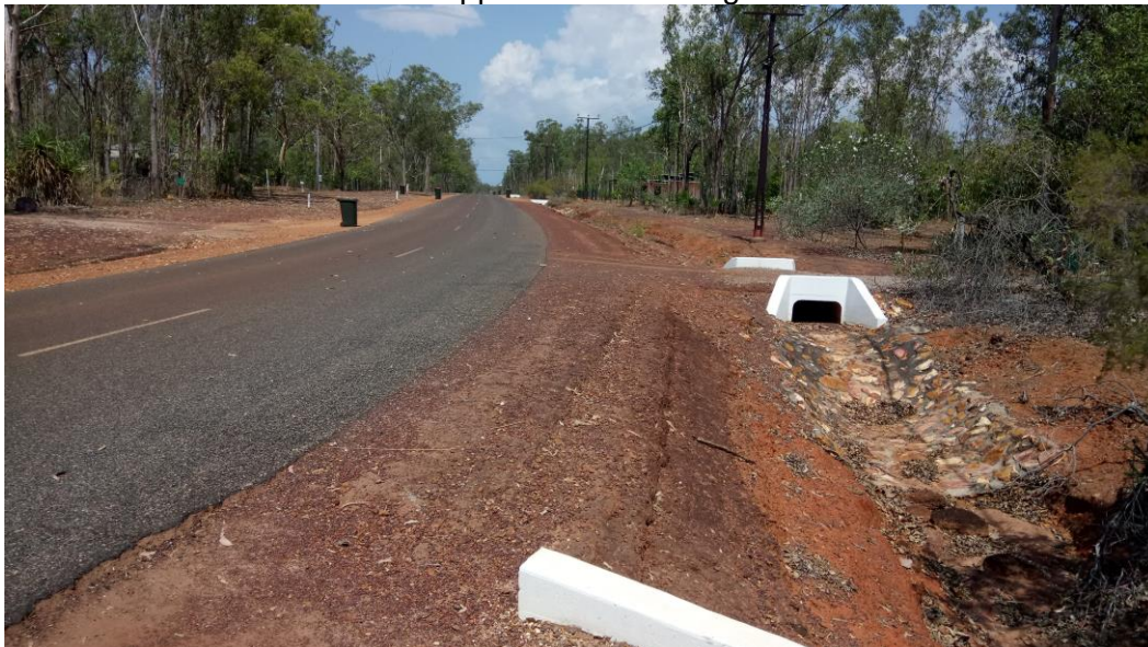
Unprotected drains and driveway culverts approximate chainage 1.1
