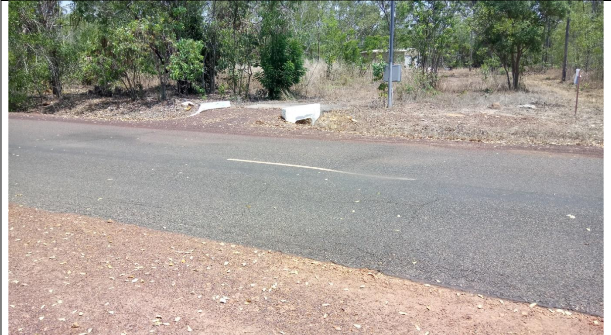
Cracking and undulation of pavement at chainage 0.25
