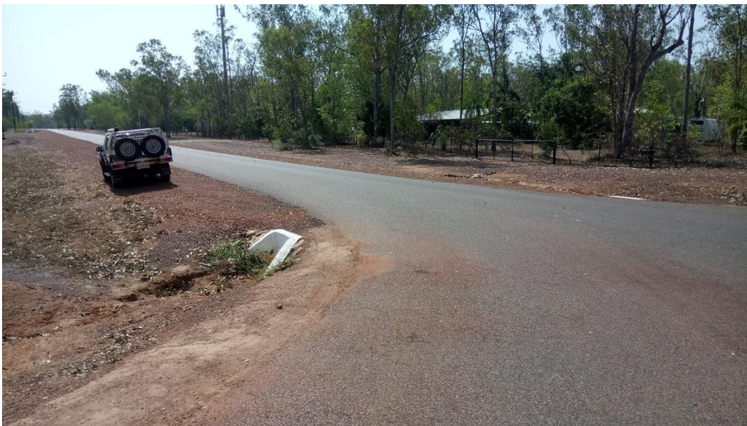
Photo: Unprotected Culvert Wagait Tower Road and Dalmeny Street Intersection
