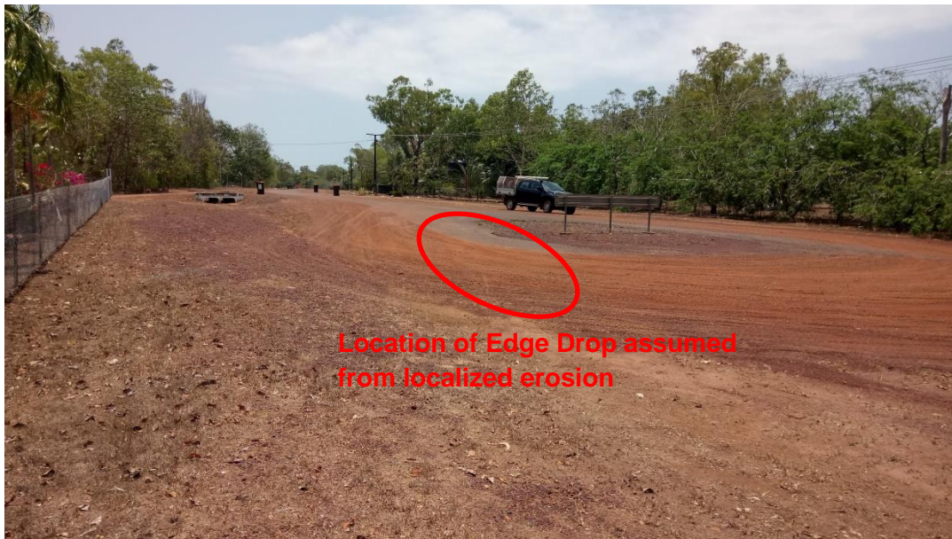
Figure 5 – Road section of maintenance concern, 105 De Lissa Drive
