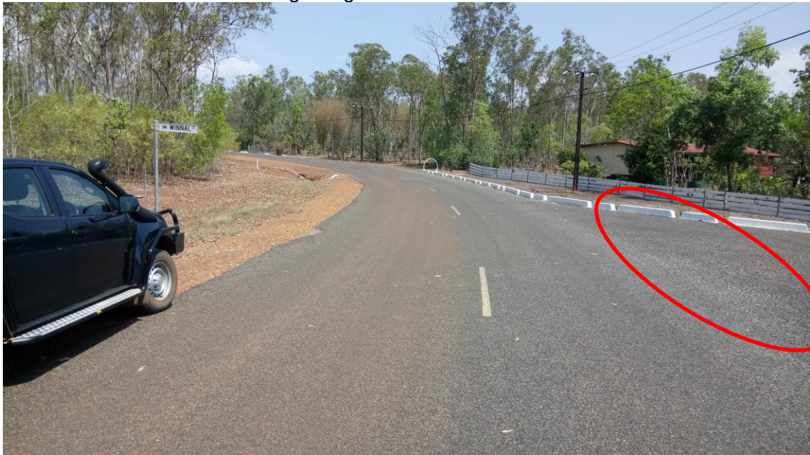
Raveling Winnal Court Intersection
