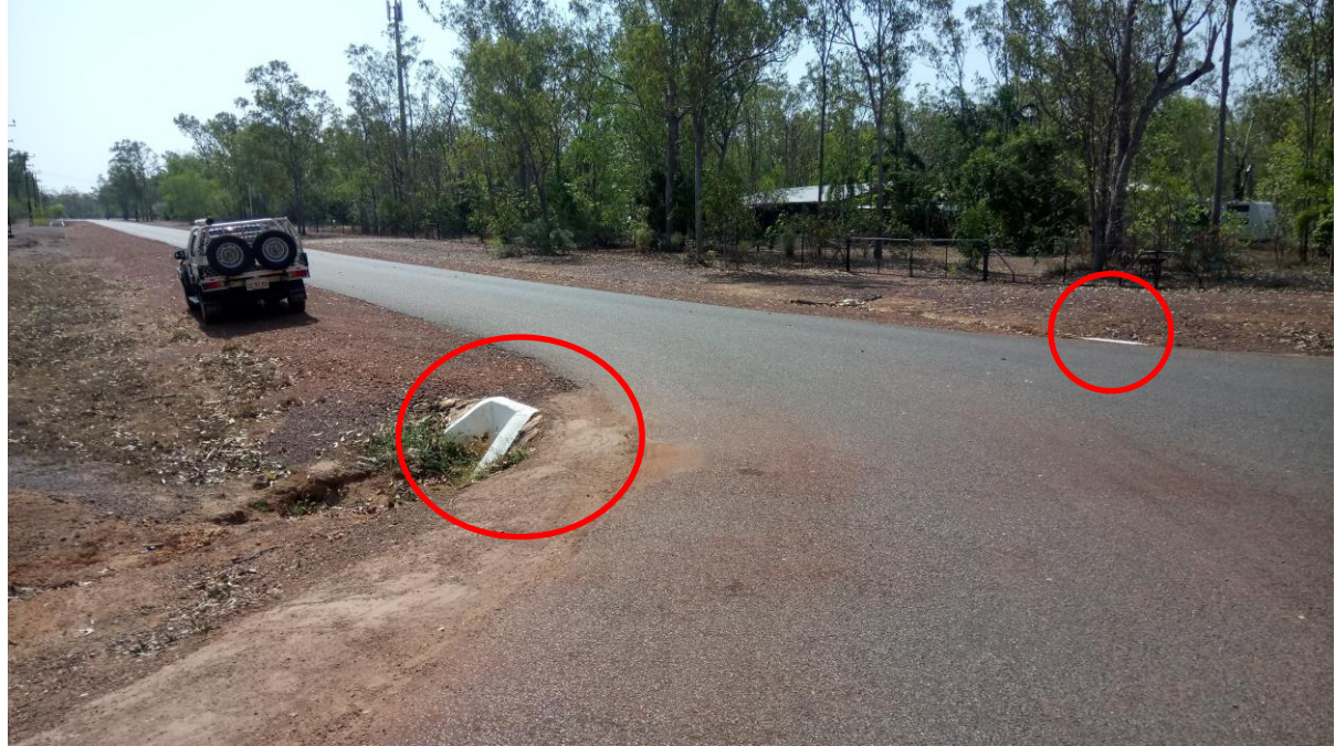
Unprotected drainage structure Wagait Tower Road
