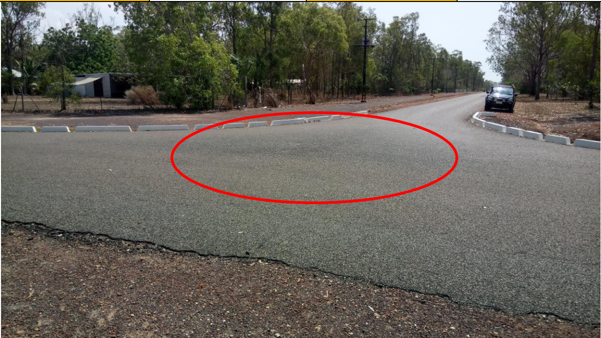
Ravelling at Erickson Crescent Intersection
