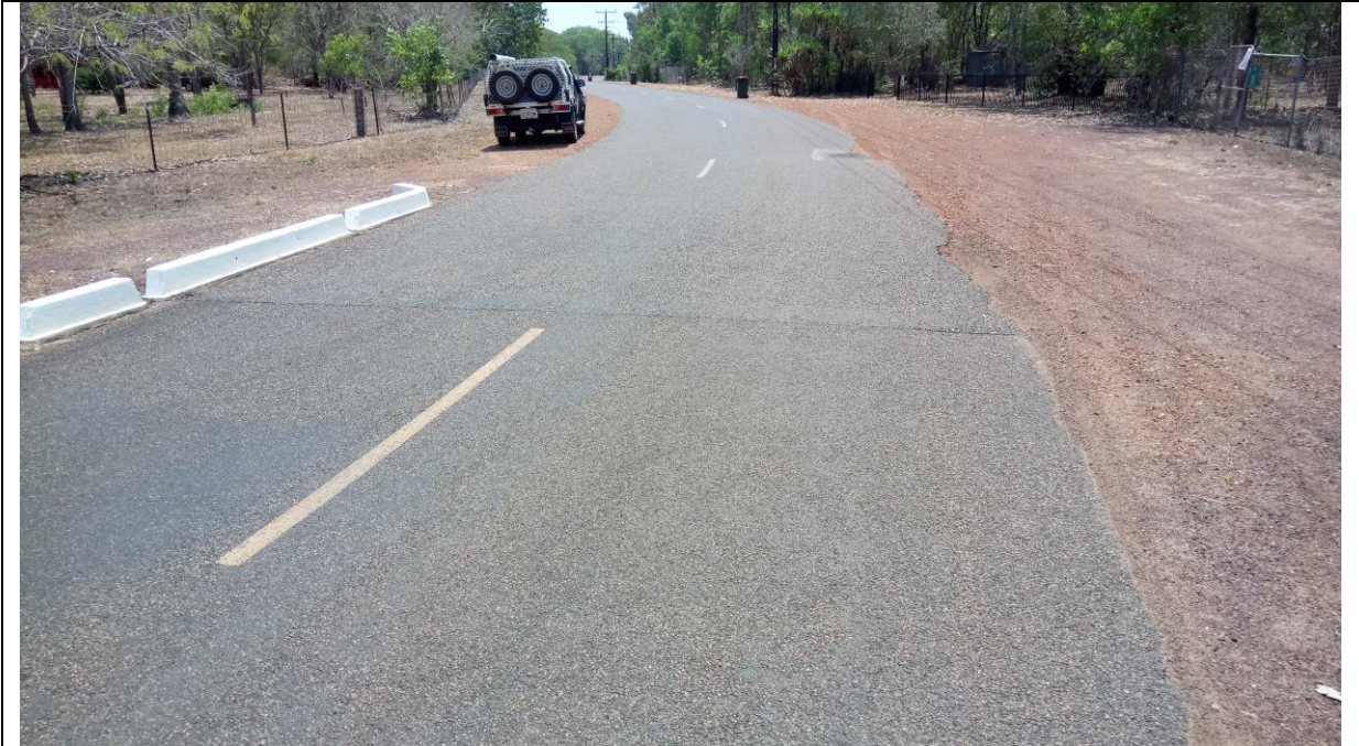
Edge break at approximate chainage 0.7
