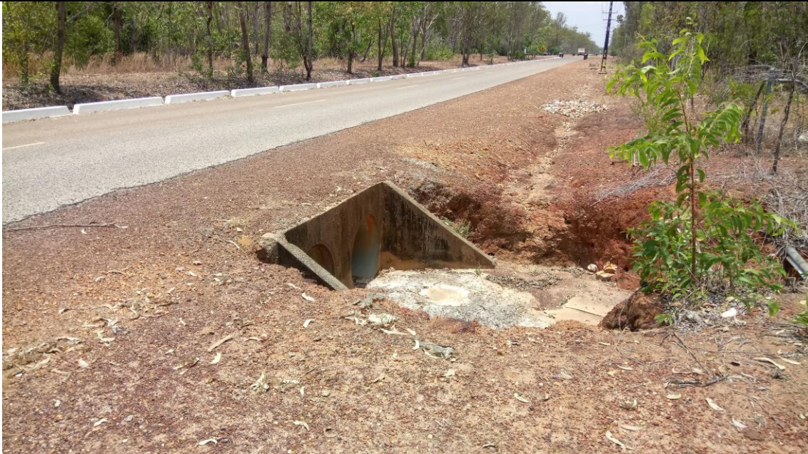
Unprotected culvert crossing at approximate chainage 1.05
