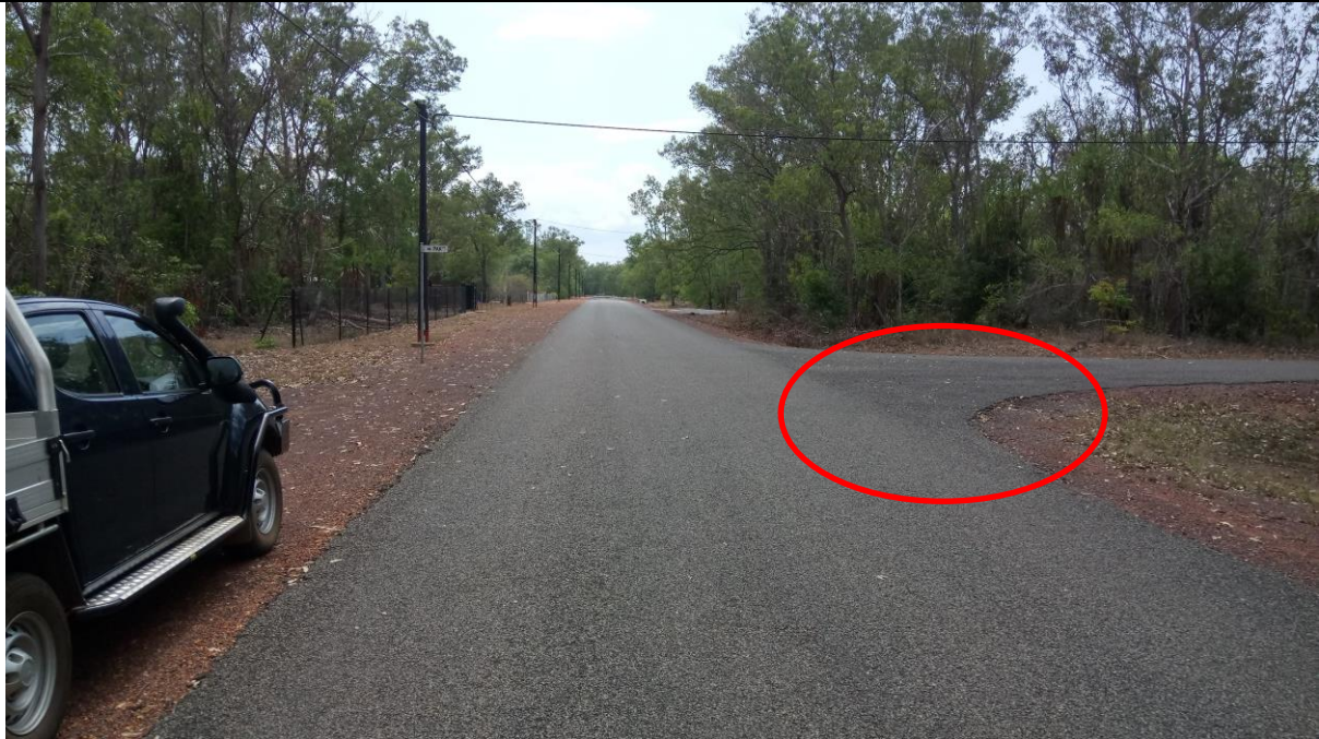
Raveling at Pak Place Intersection
