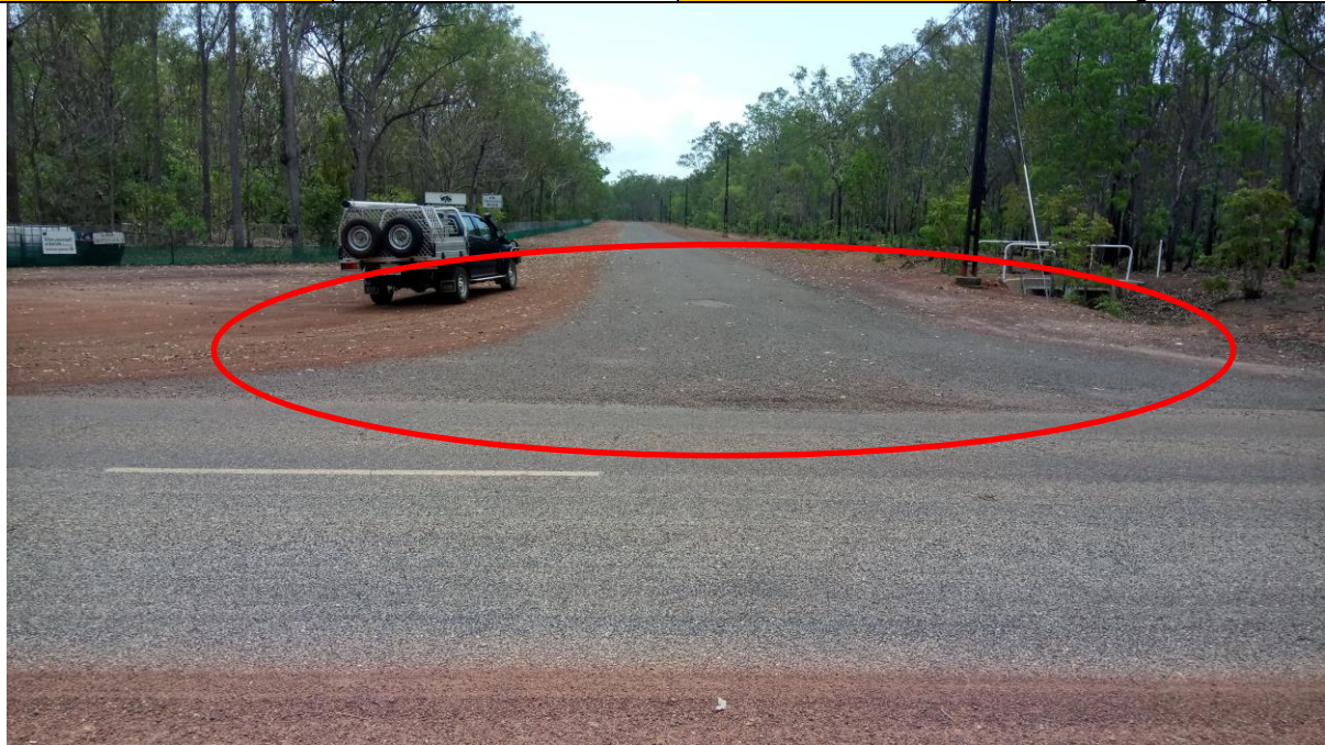
Raveling at Wagait Tower Road Intersection
