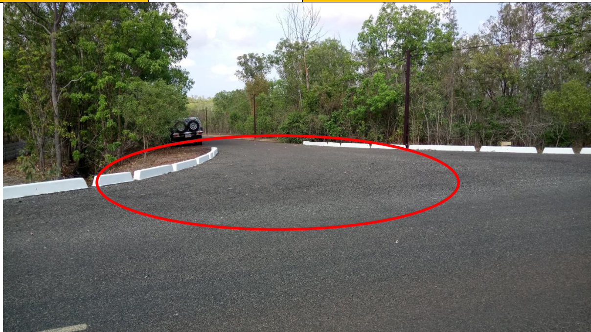
Raveling at Erickson Crescent Intersection
