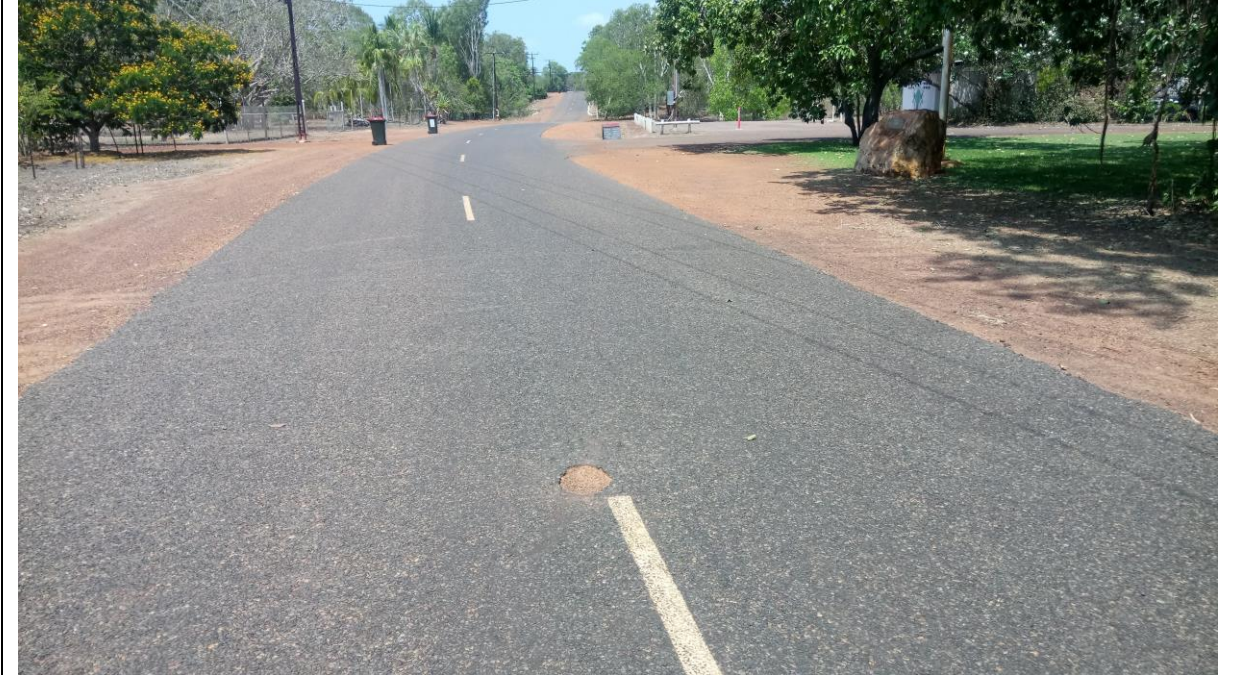
Pot hole forming at Chainage 1.05
