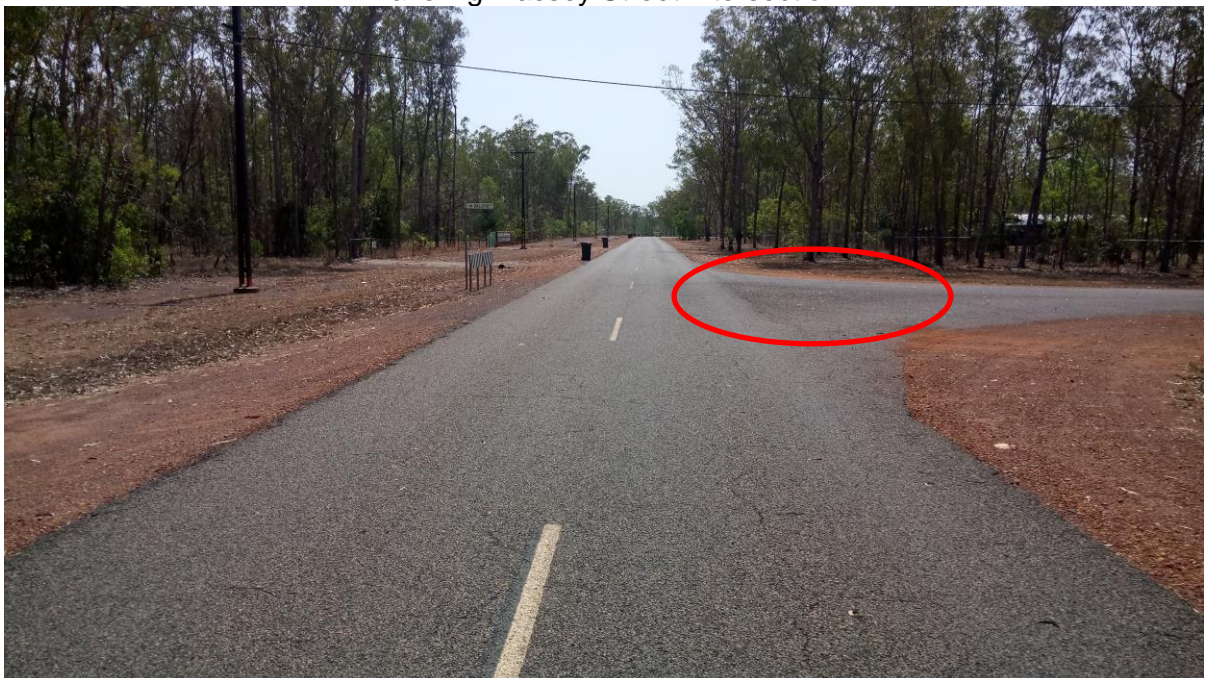
Raveling Baluria Road Intersection
