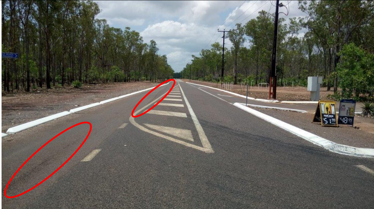
Cracking at approximate chainage 0.1
