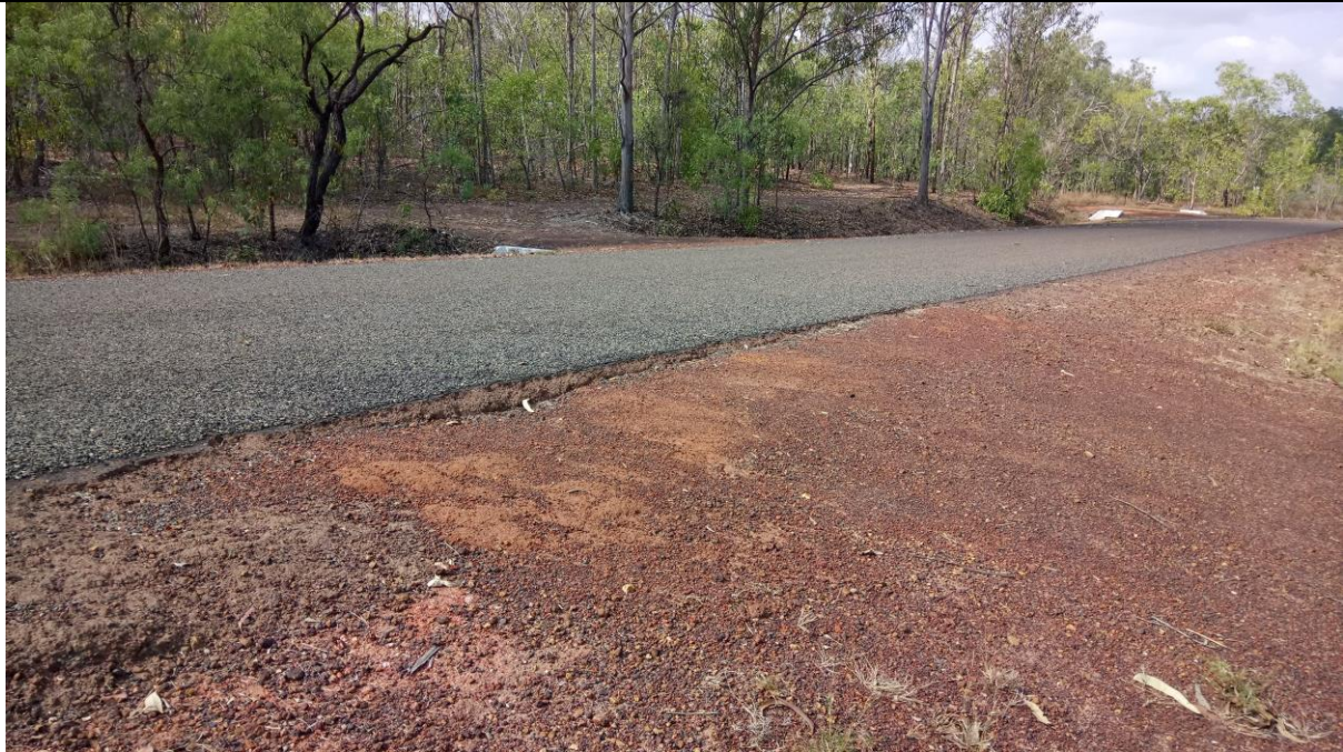
Edge drop at driveway
