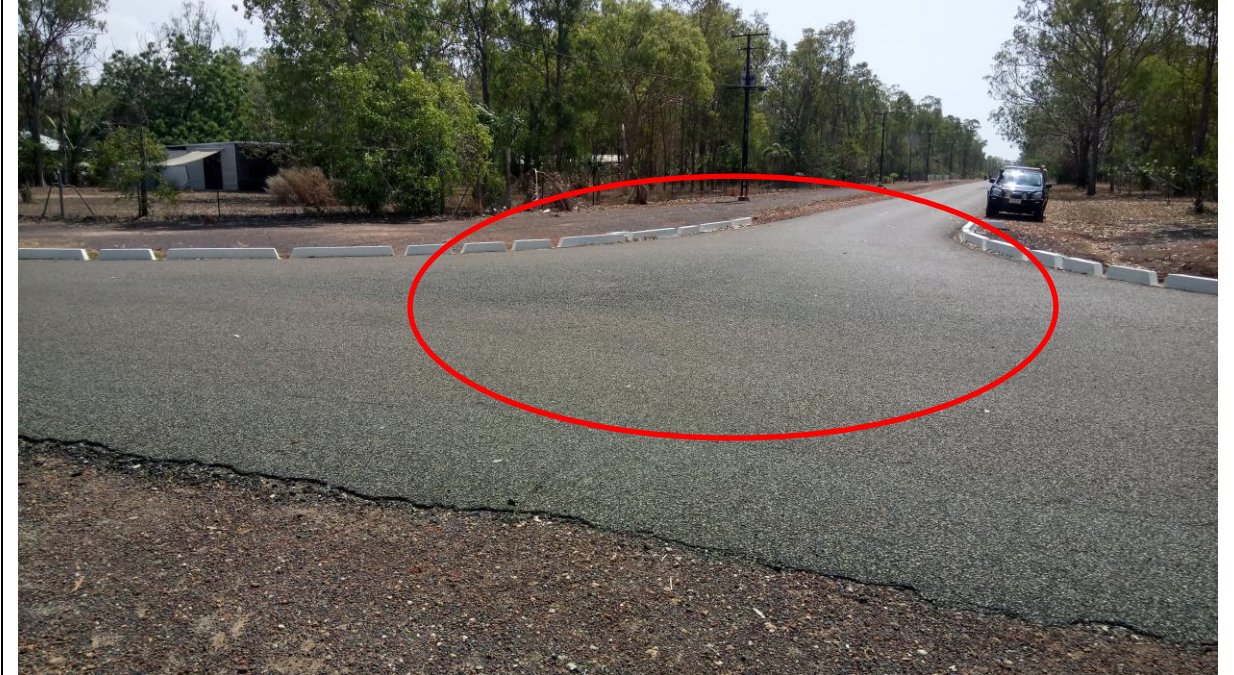
Ravelling Brisbane Street Intersection
