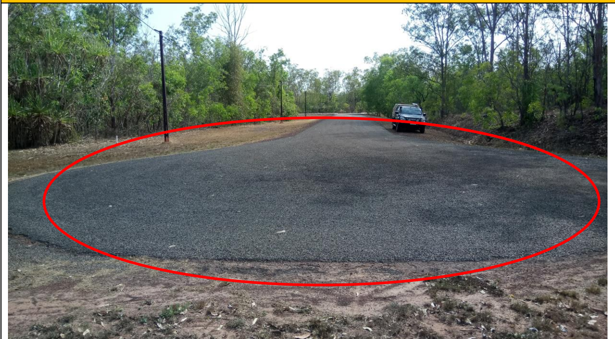
Raveling at Cul-de-sac
