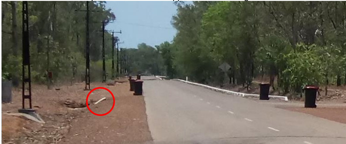
Unprotected culvert at approximate chainage 0.75
