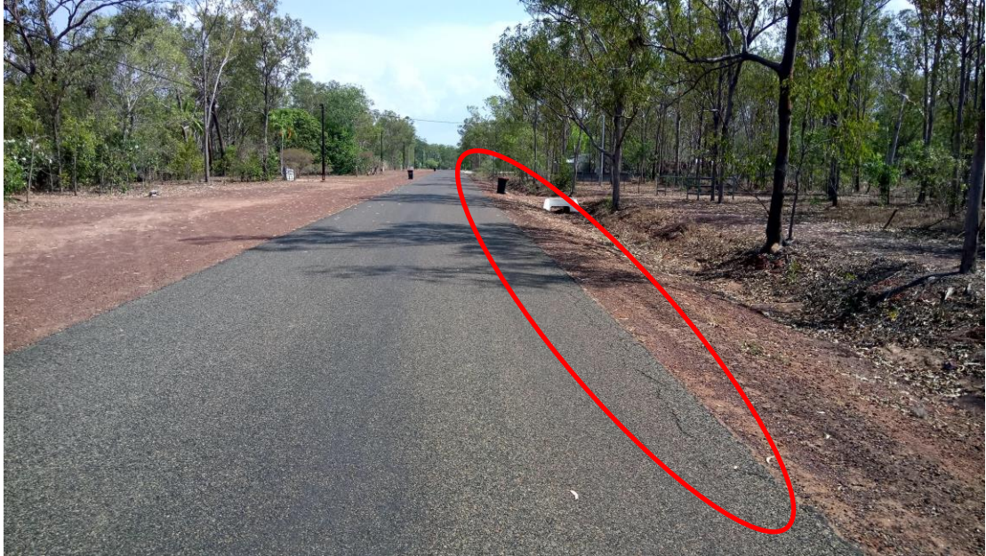
Cracking between CH0.4-CH0.5
