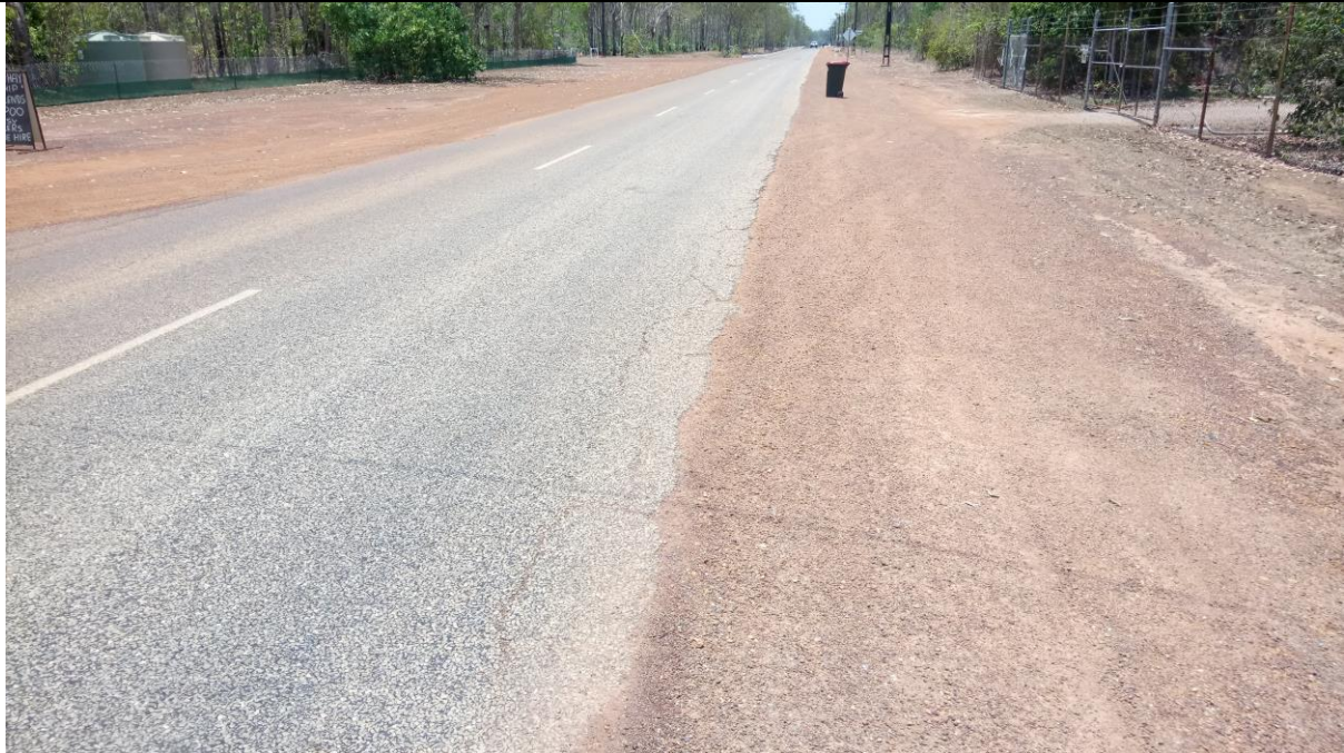
Edge breaks and cracking at approximate chainage 0.6
