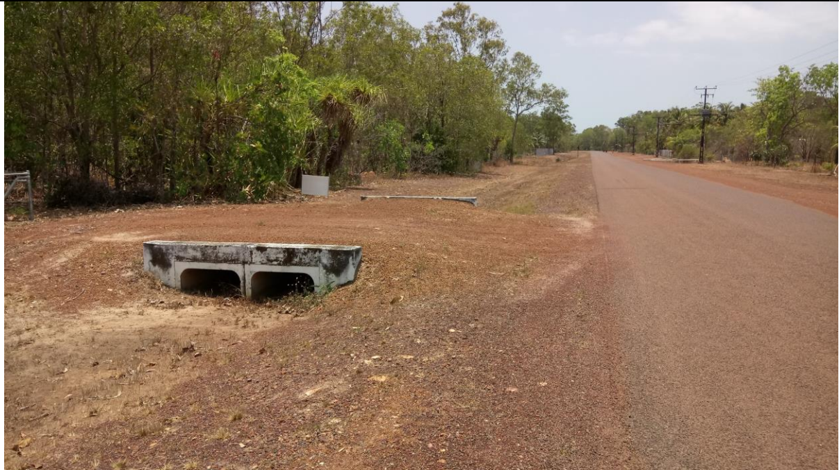
Unprotected driveway culvert approximate chainage 0.95
