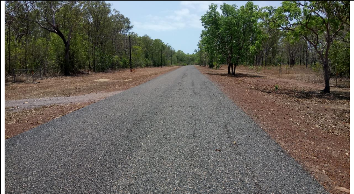
Raveling at approximate chainage 0.4
