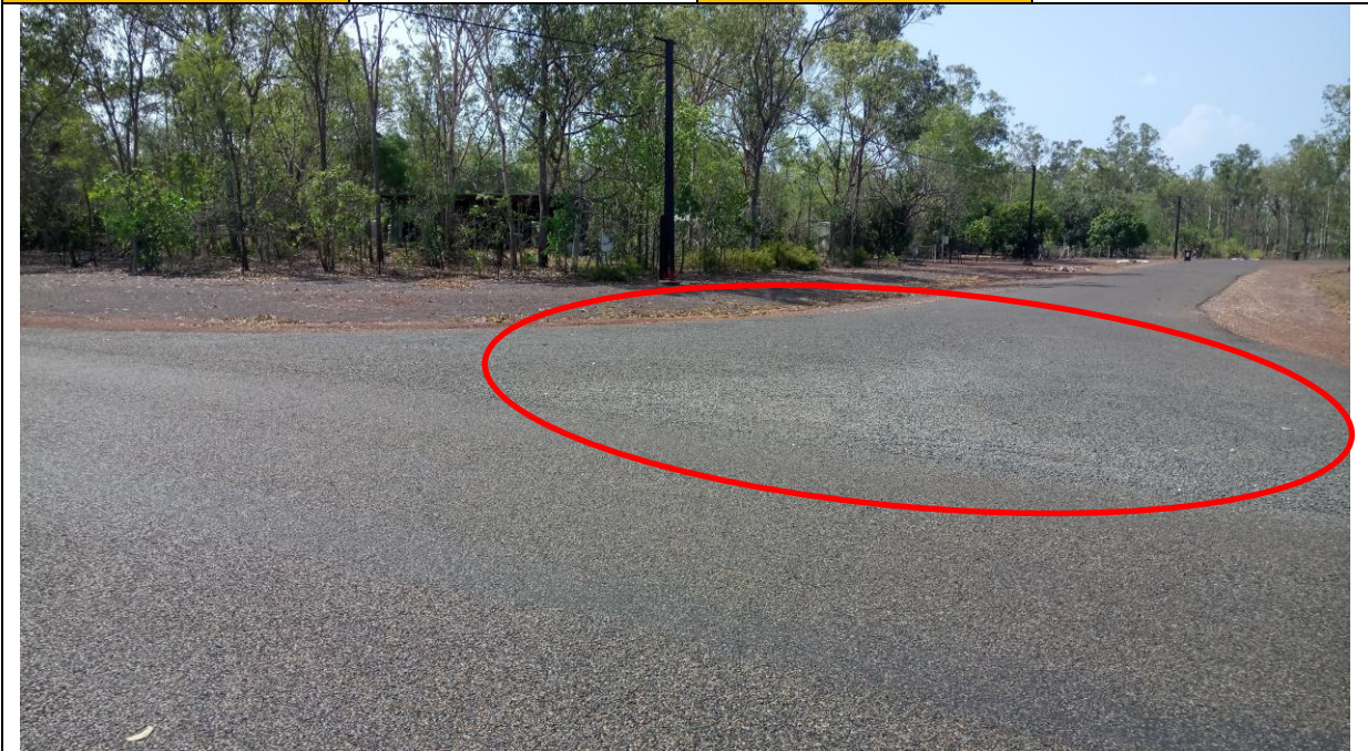
Ravelling at Head Crescent
