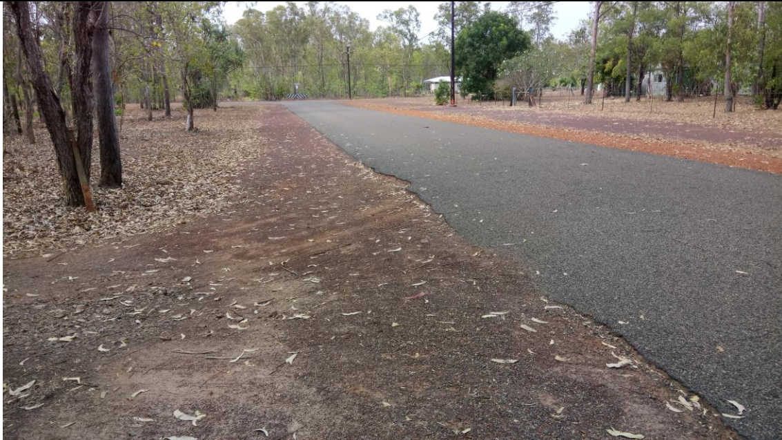
Edge break approximate chainage 0.35
