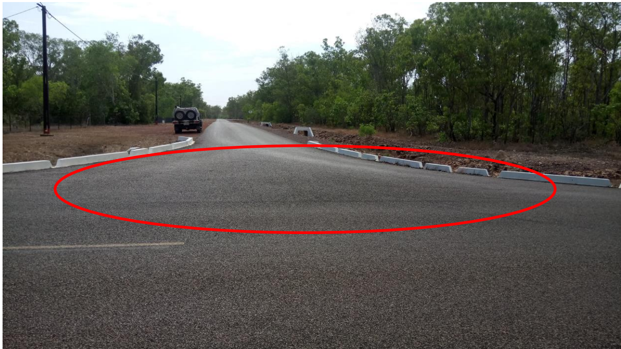
Raveling at Erickson Intersection
