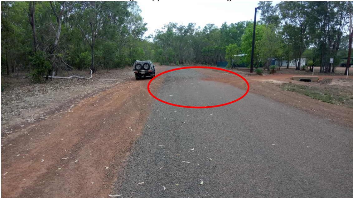
Raveling at recreational centre entrance
