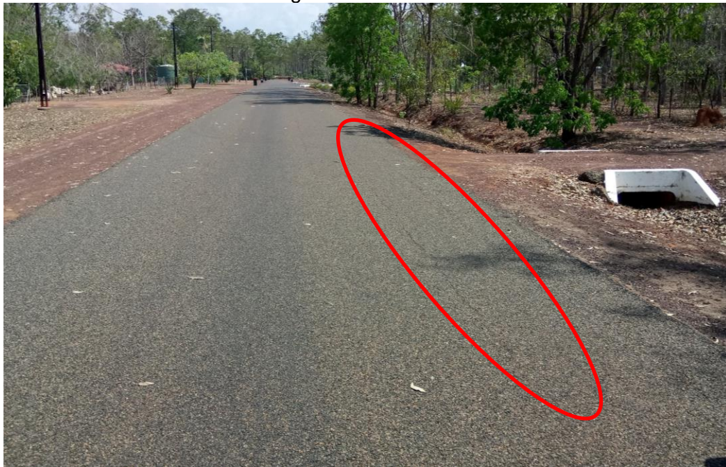
Cracking between CH0.1-CH0.2
