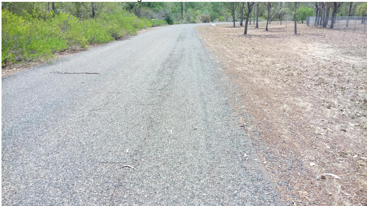
Raveling at approximate chainage 0.25
