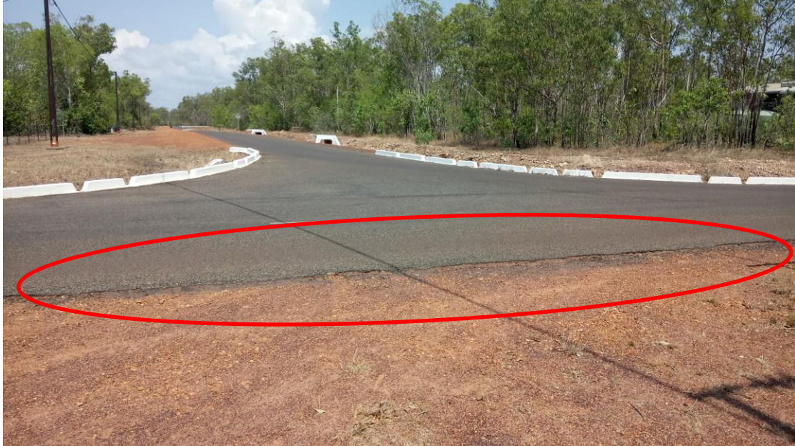
Edge drop approximate chainage 0.4
