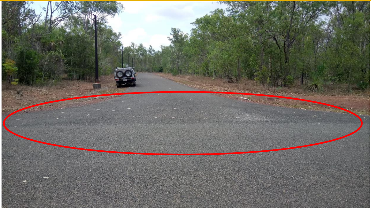
Raveling at Uhr Road Intersection
