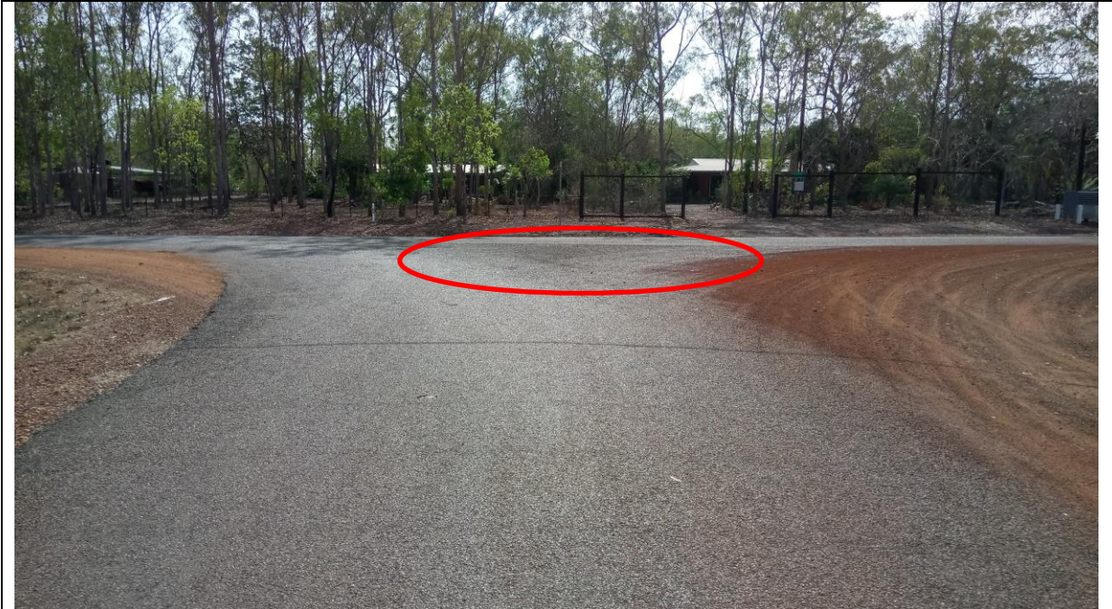
Raveling at Cul-de-sac
