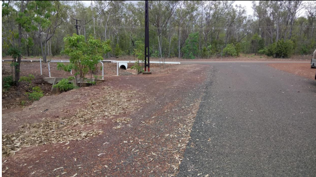
Unprotected drainage structure adjacent to Wagait Tower Road
