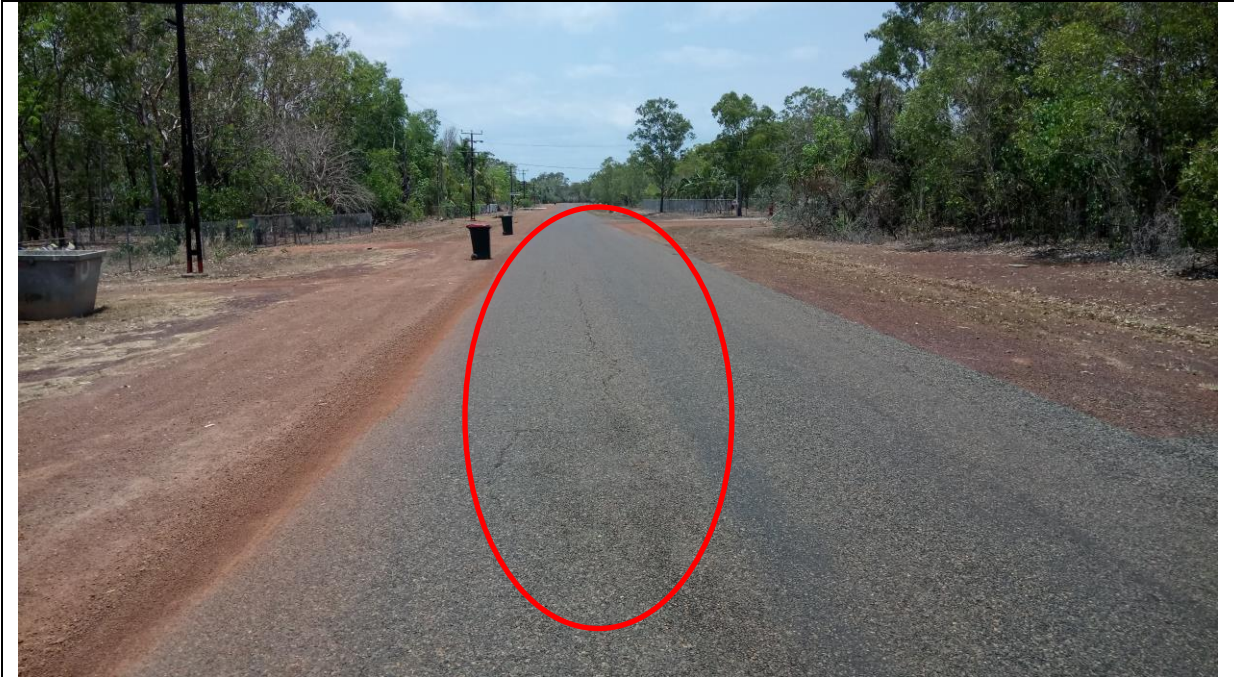
Pavement cracking approximate chainage 0.2
