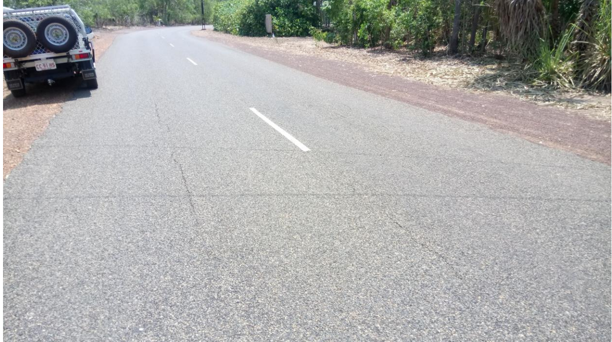
Longitudinal cracking at approximate chainage 0.3
