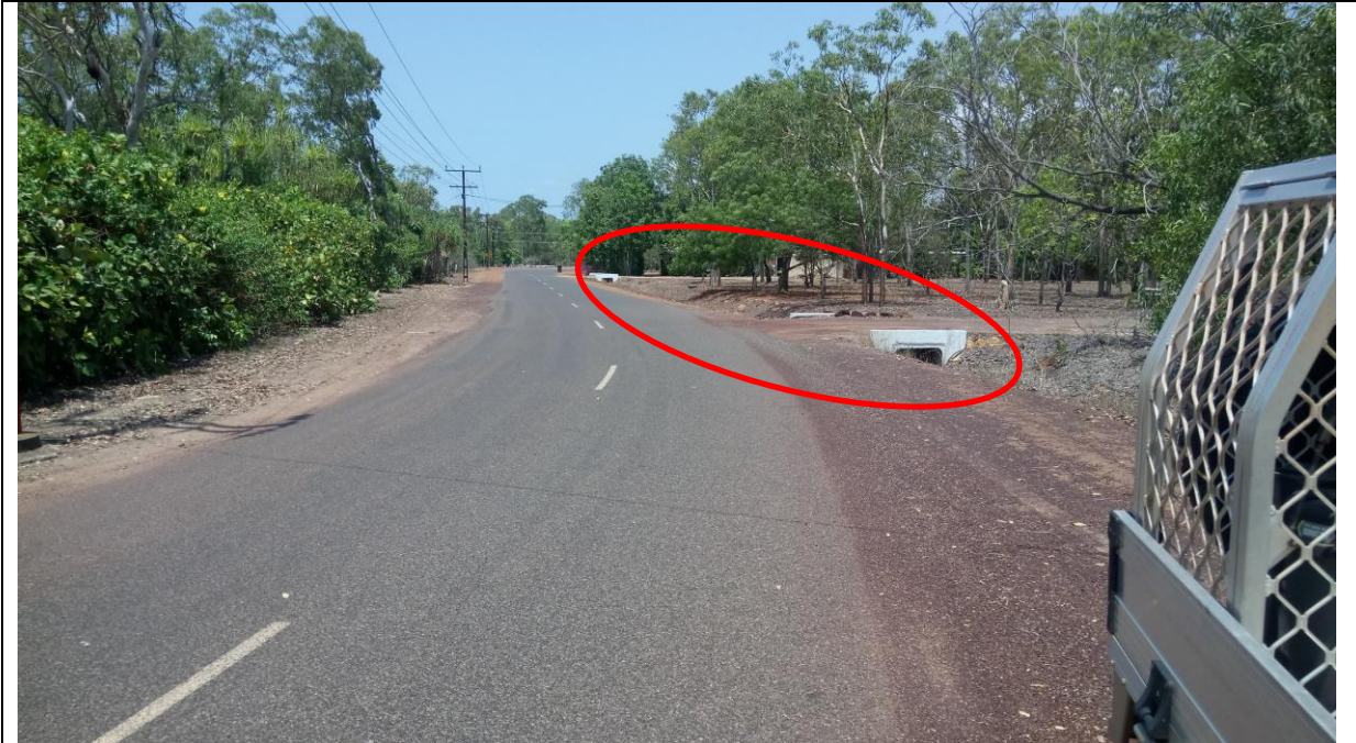
Unprotected driveway culverts approximate chainage 0.3
