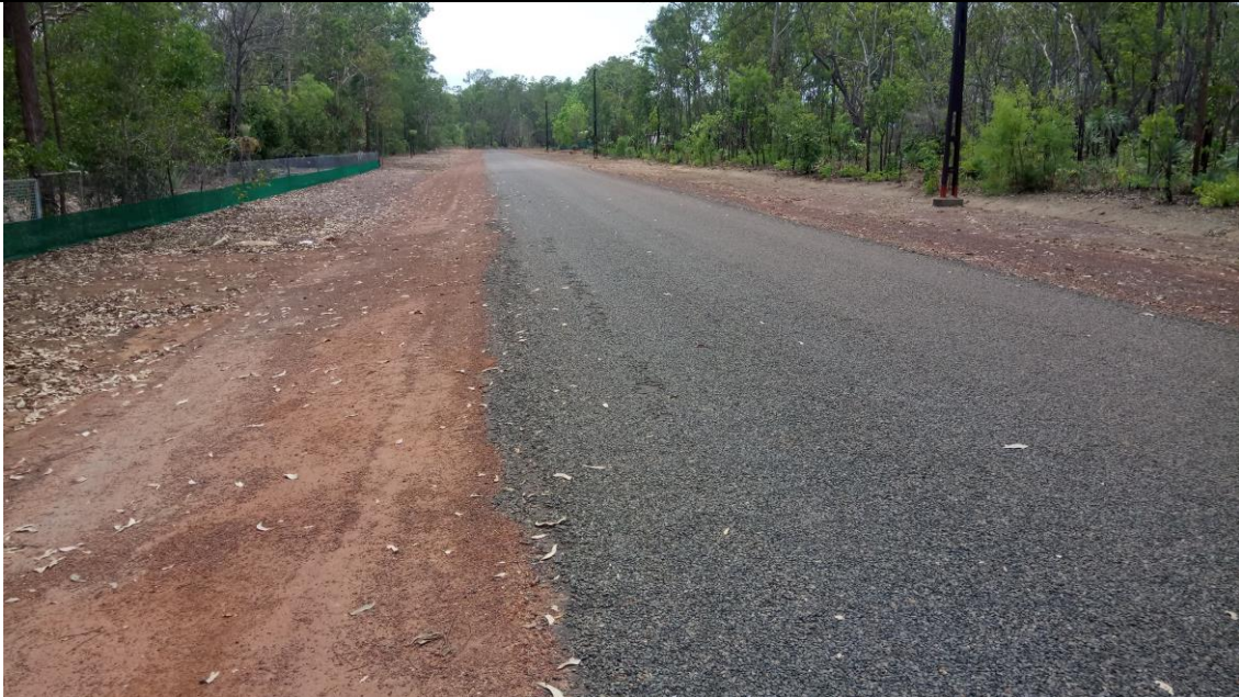
Raveling at approximate chainage 0.15
