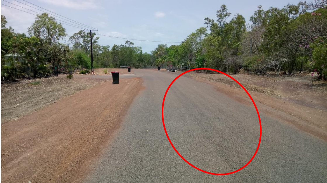
Appearance of potential raveling at approximate chainage 0.8
