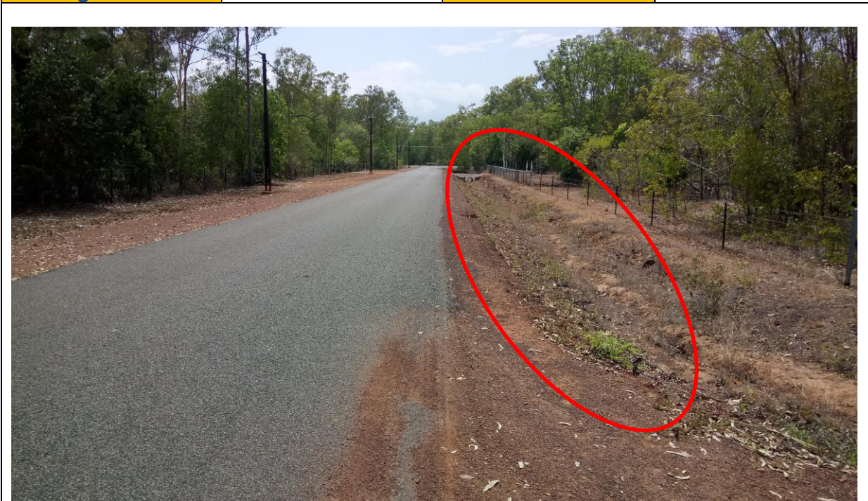
Unprotected drainage structure and driveway culverts approximate chainage 0.4
