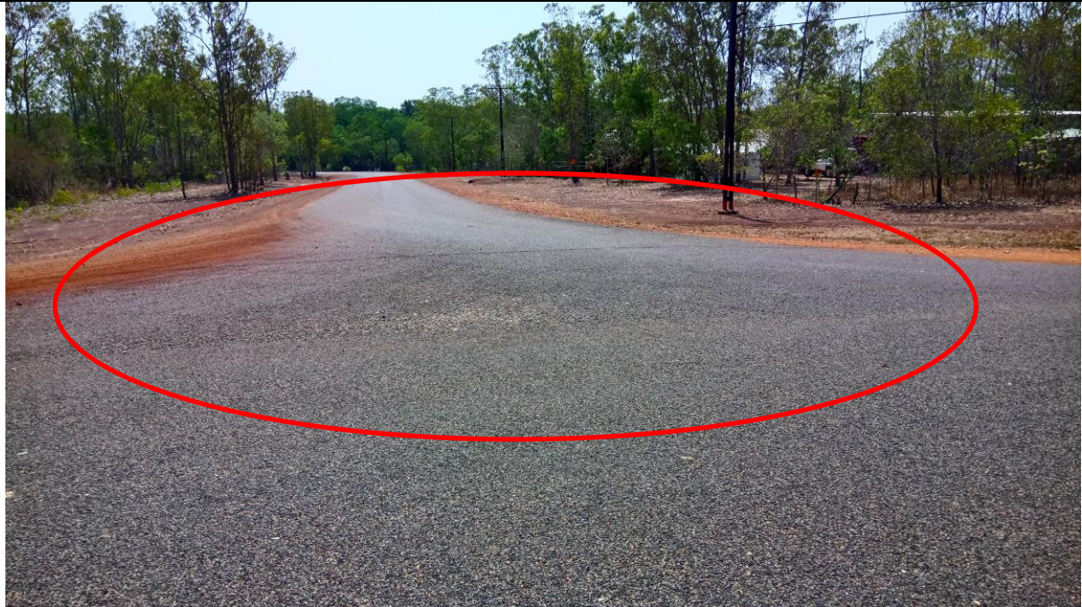
Raveling Vangemann Street Intersection
