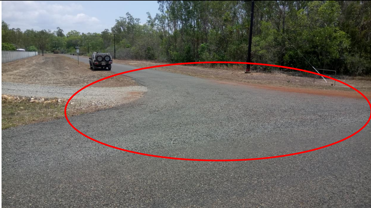
Raveling at De Lissa Road Intersection
