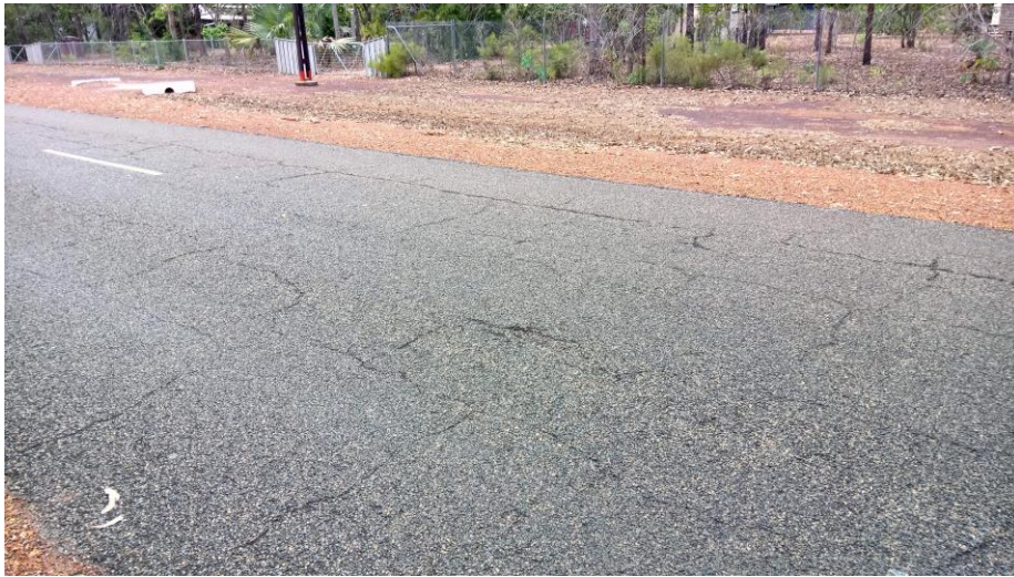
Photo: Erickson Crescent Pavement Cracking
