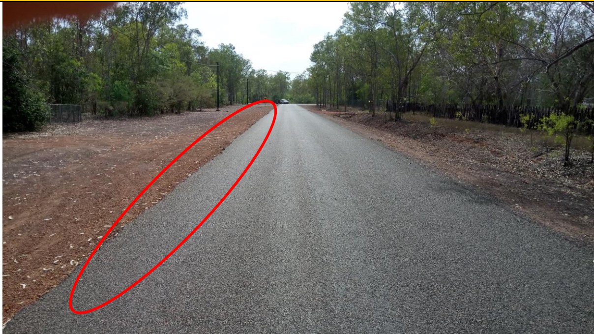
Edge drop approximate chainage 0.3
