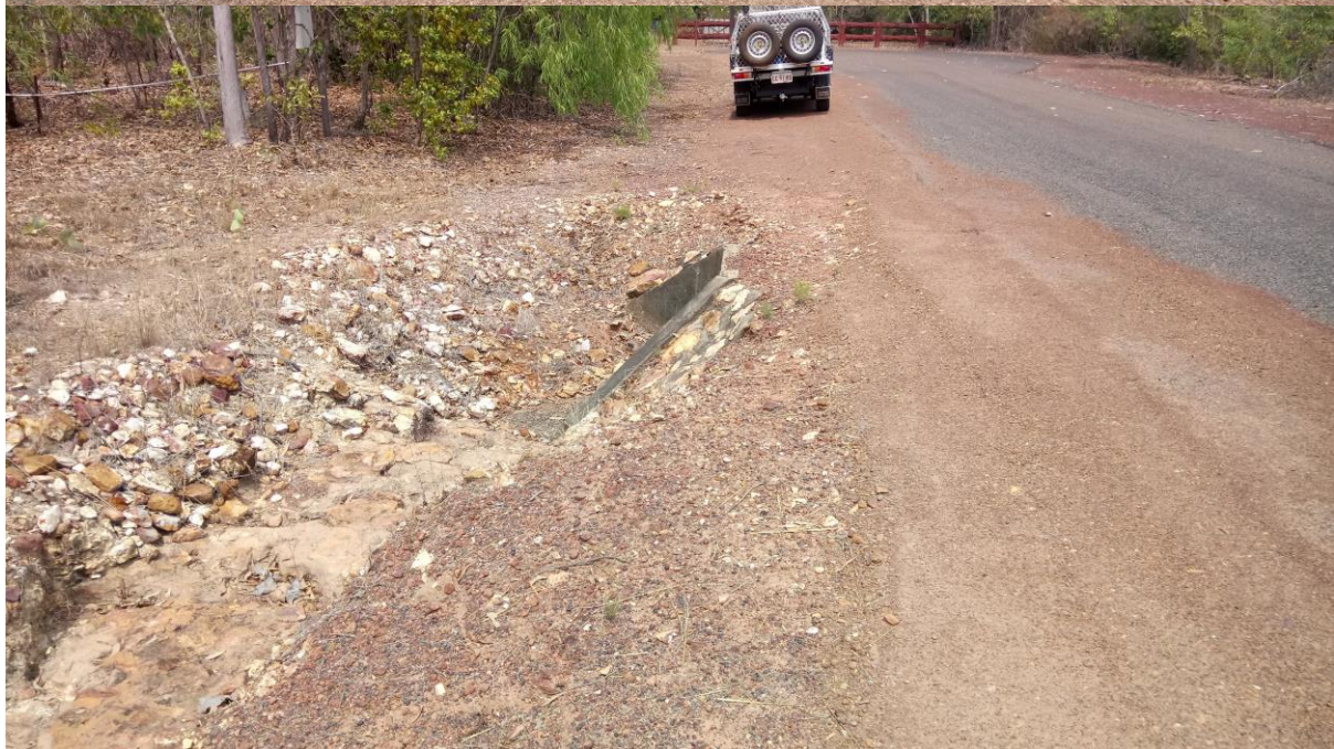
Unprotected culvert crossing at Dillon Place Intersection
