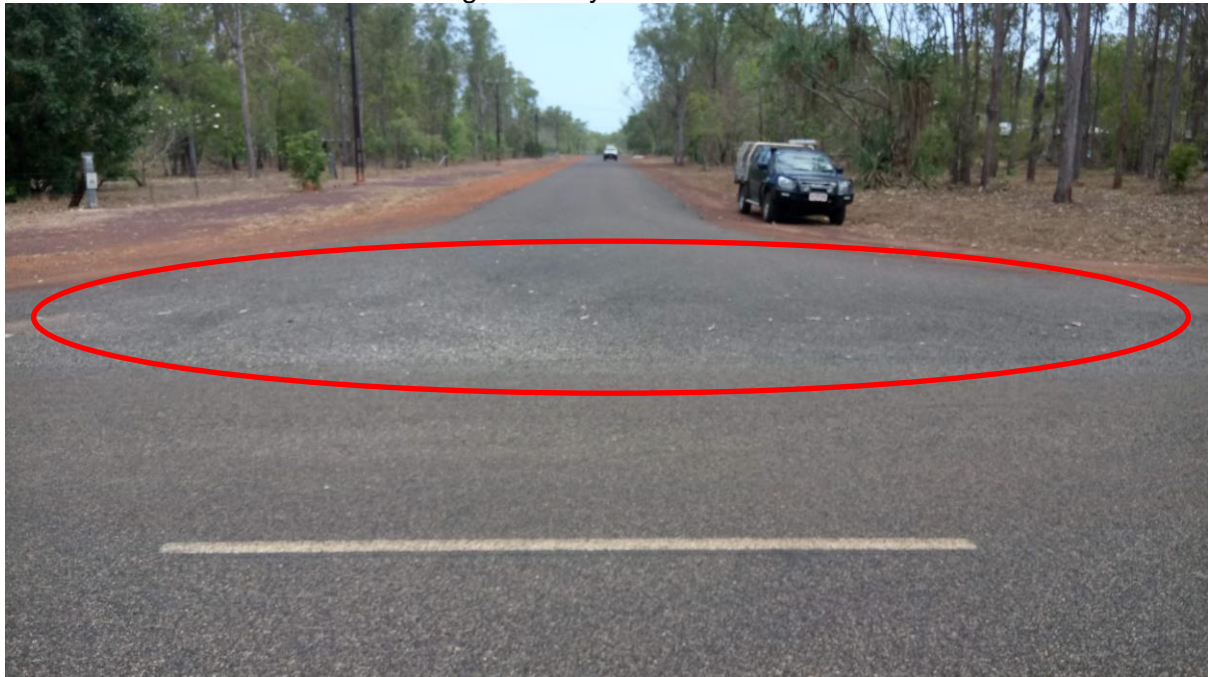
Raveling at Erickson Crescent Intersection
