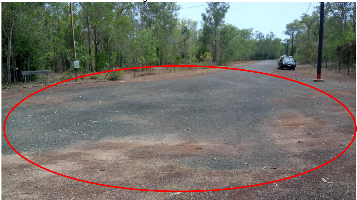
Raveling at Cul-de-sac
