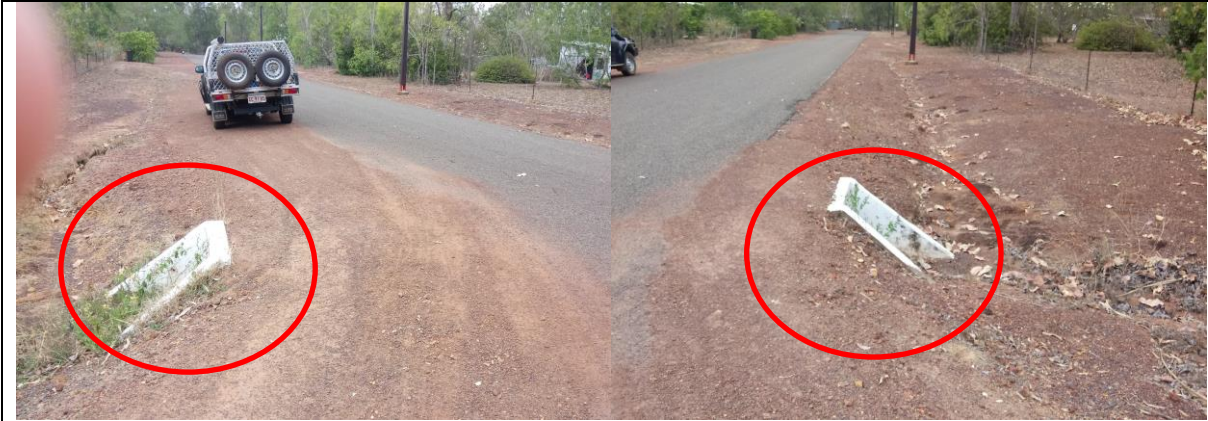
Unprotected culvert at Uhr Road intersection
