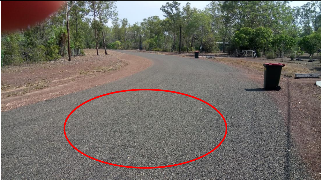
Cracking approximate chainage 0.1
