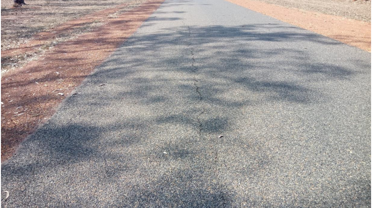
Longitudinal Cracking between Erickson Crescent and Dalmeny Road
