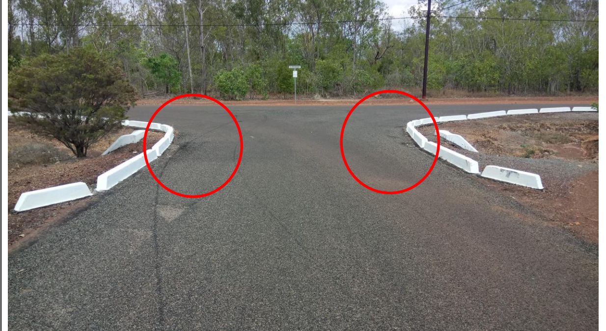
Raveling at Erickson Crescent
