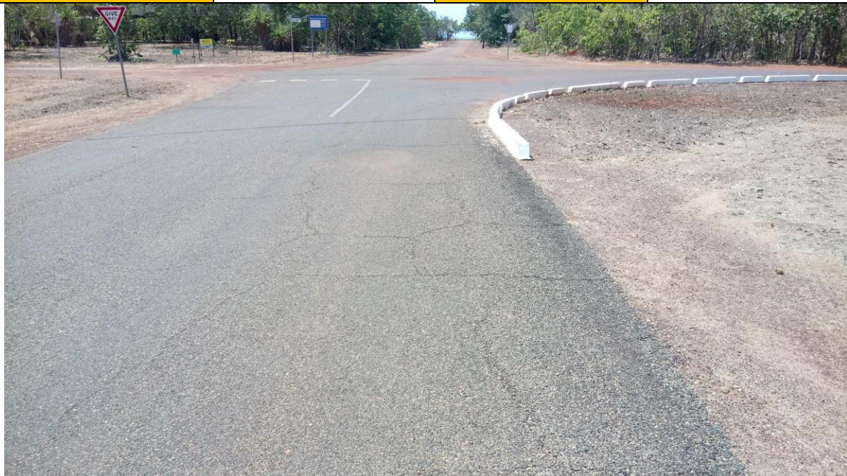
Cracking Cox Drive Intersection
