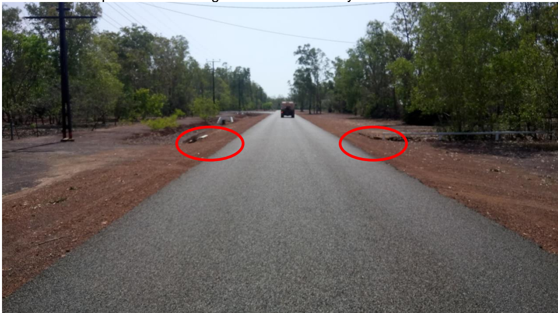
Unprotected Drainage Structure approximate chainage 0.15
