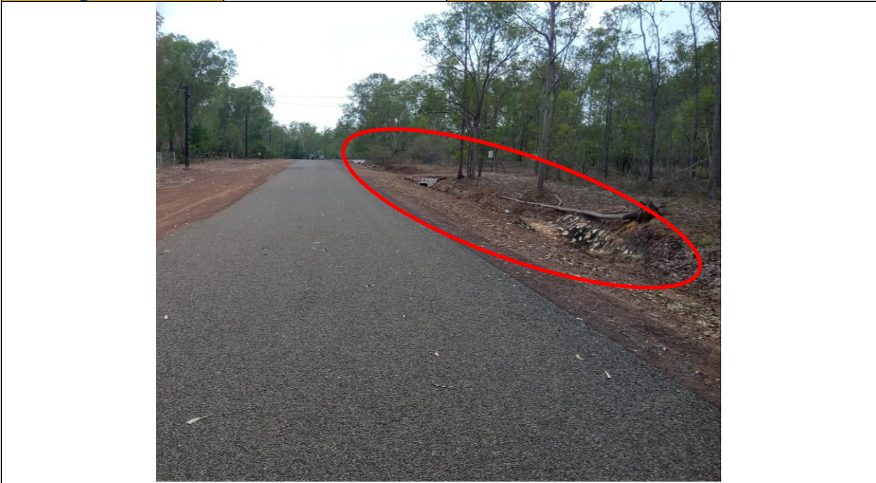
Unprotected drainage structures along southern edge of roadway
