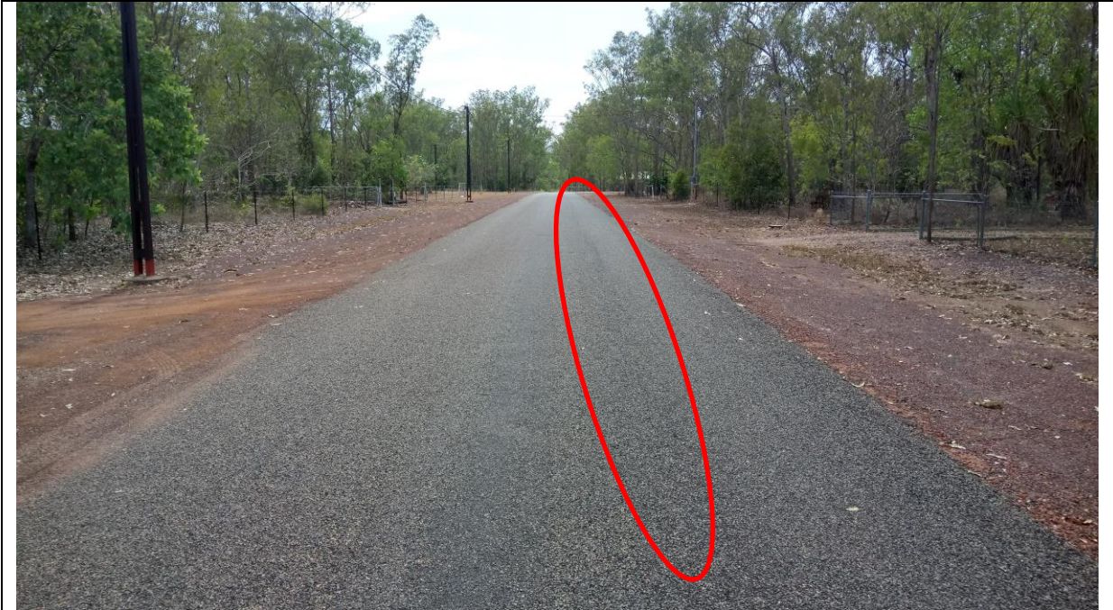
Pavement cracking at approximate chainage 0.1
