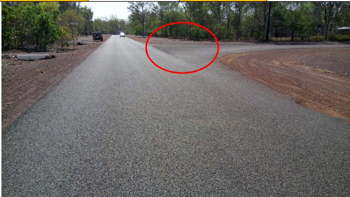
Raveling at Dalmeny Street Intersection
