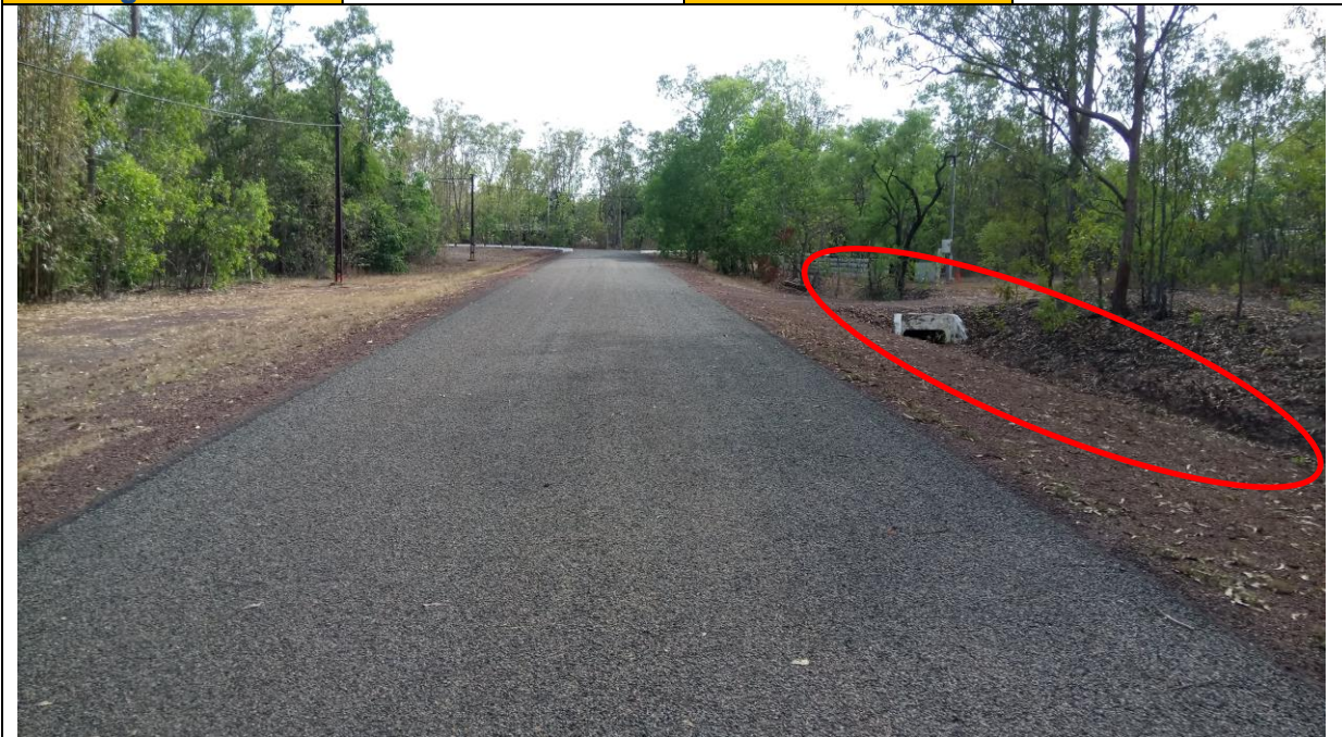
Unprotected drain and driveway culvert at approximate chainage 0.05
