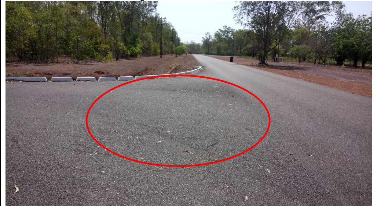
Ravelling at Dalmeny Street Intersection
