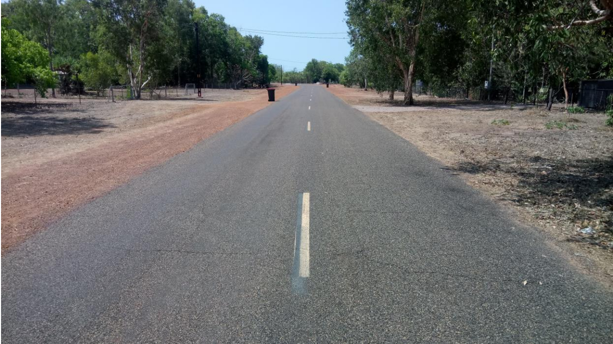
Cracking approximate chainage 0.2
