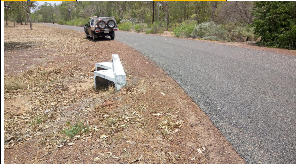
Unprotected culvert at approximate chainage 0.2
