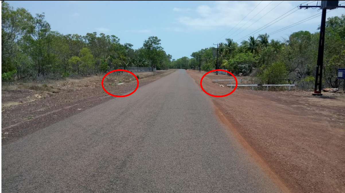
Unprotected drainage structure approximate chainage 0.45
