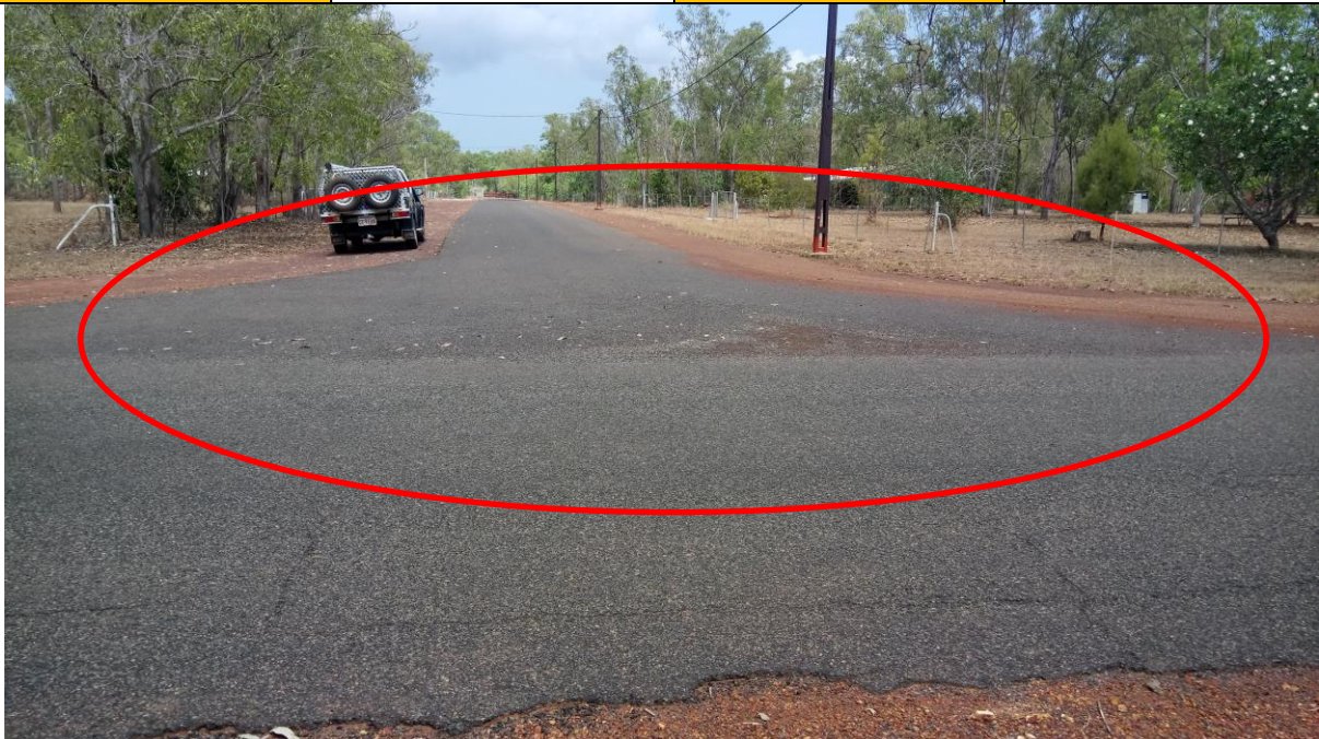
Raveling at Baluria Road Intersection
