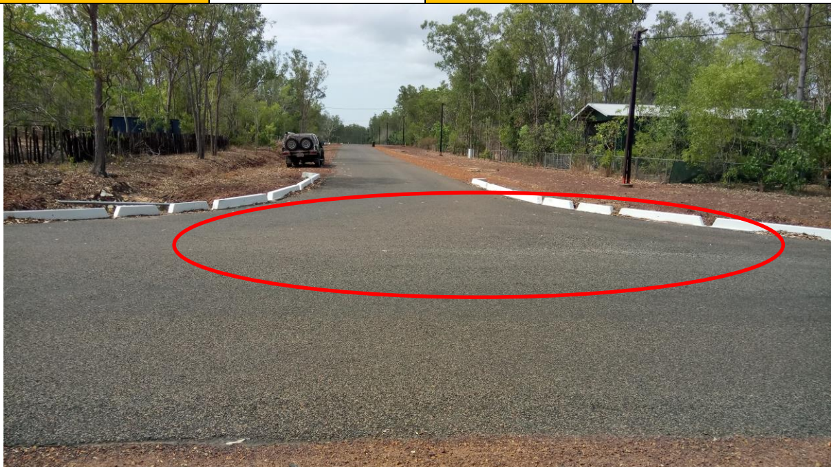
Raveling at Sachse Street Intersection
