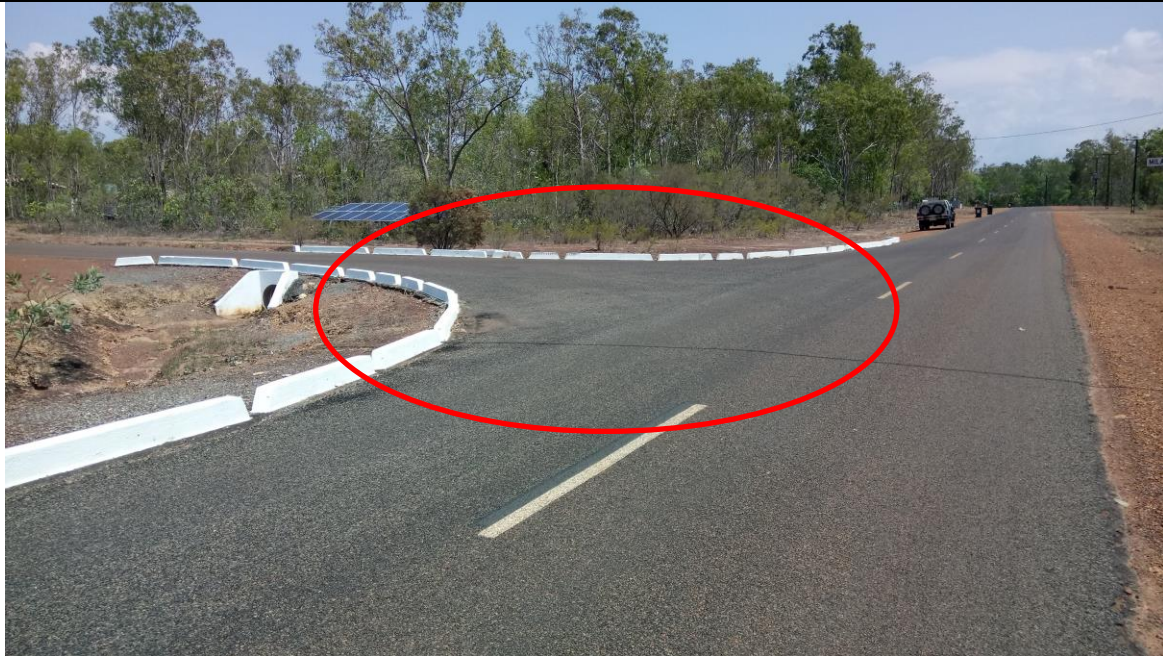
Raveling Milady Street Intersection
