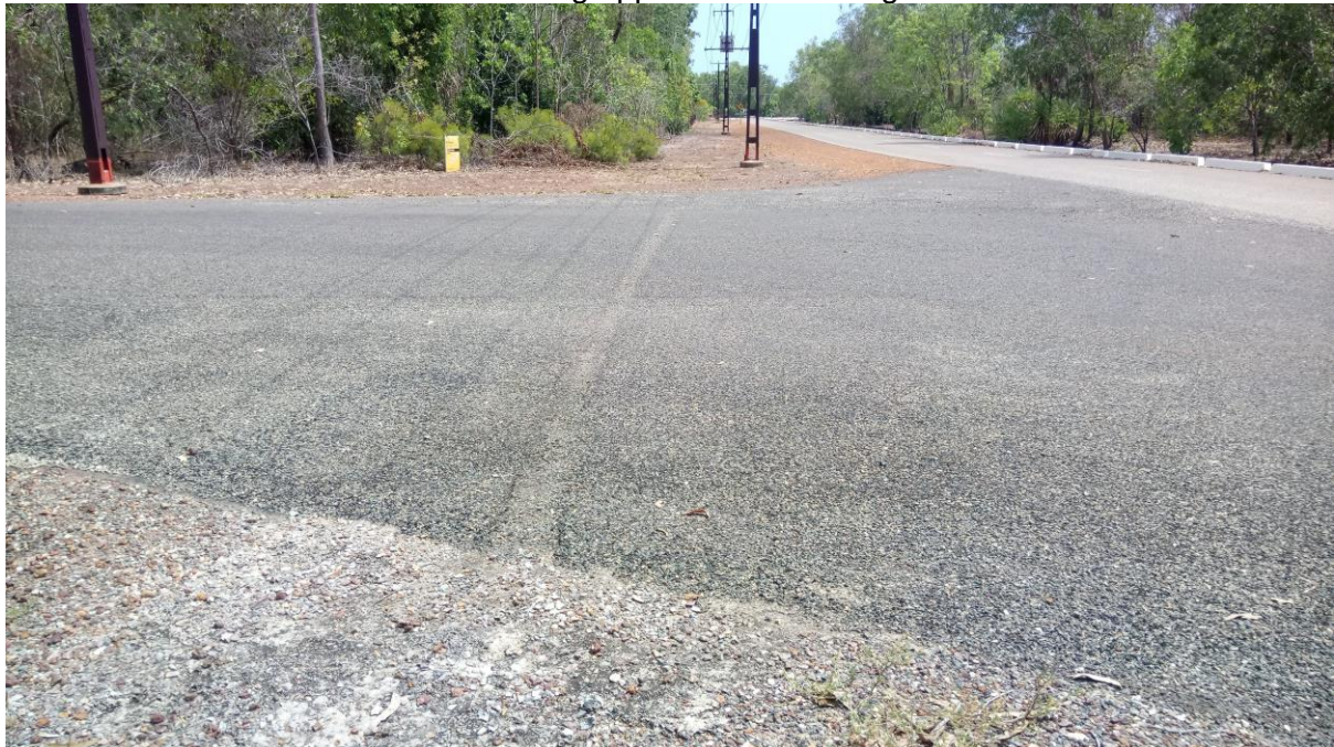
Service crossing Wagait Tower Road Intersection
