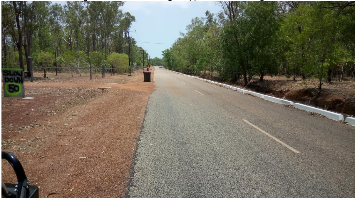
Edge breaks at approximate chainage 1.0
