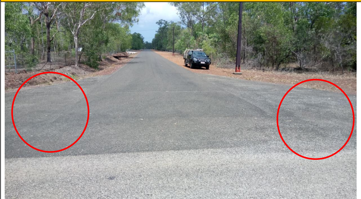
Raveling at Wagait Tower Road
