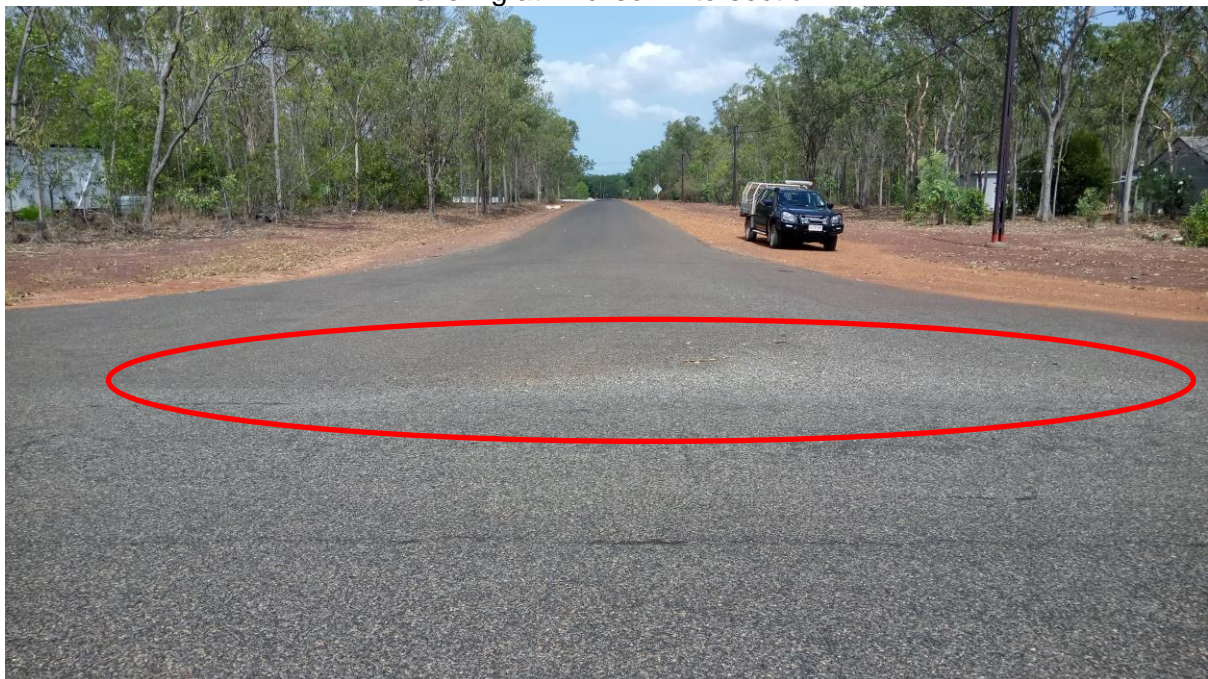
Raveling at Baluria Road Intersection
