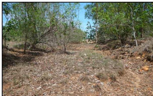
Drain from De Lissa Dve between Lots 12 & 13 to beach. Potential salt marsh mosquito breeding site. Sediment build-up in lower reaches, similar to other drains at Wagait Beach.
