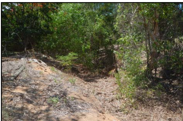
Wagait Trower Rd drain to beach. Potential salt marsh mosquito breeding site.
